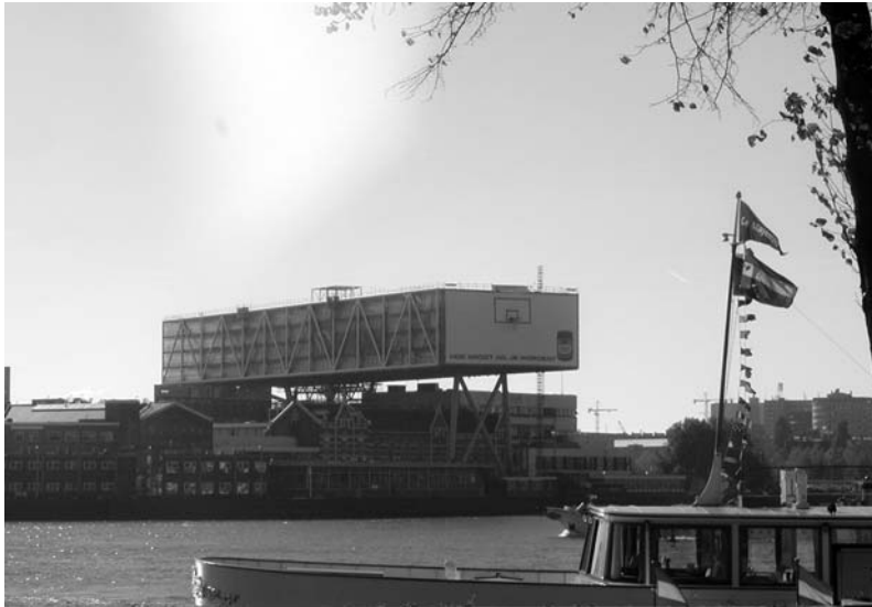
Figure 11.14 Feyenoord, 'De Brug' with a new office structure under construction by DURA-Vermeer.
