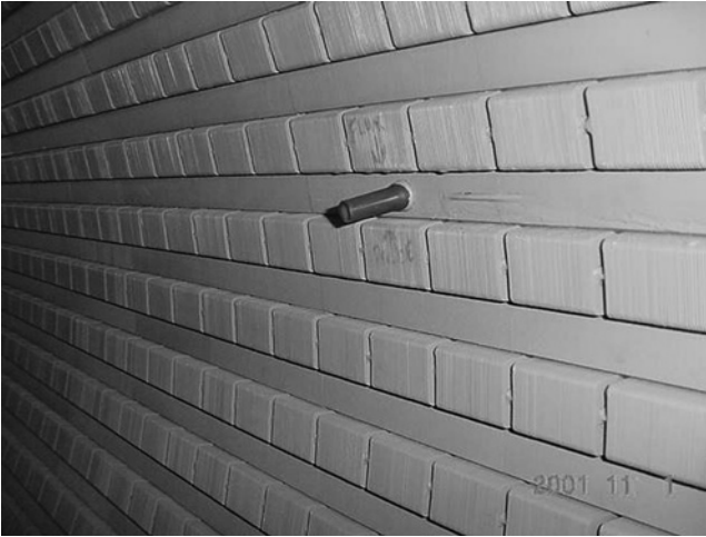
Figure 16.8 Flux probe mounted in generator stator.
