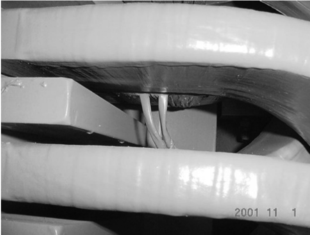
Figure 16.10 RTD mounted in generator stator between top and bottom coils.
