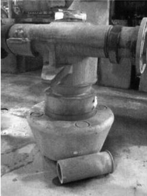
Figure 3.13 Vertical spindle coal mill roll assembly.
