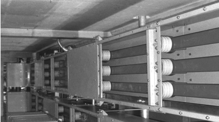
Figure 14.8b Non-segregated phase bus duct. Source: Reproduced with permission of Crown Electric Engineering and Manufacturing LLC.
