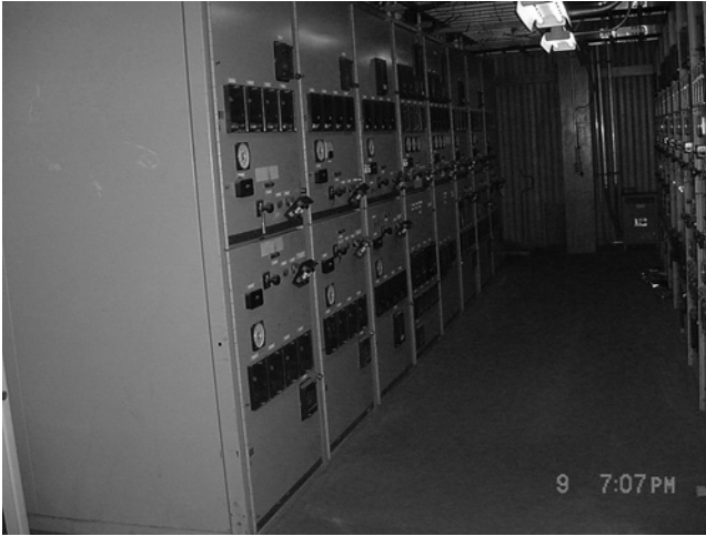
Figure 19.1 13.8 kV switchgear lineup.
