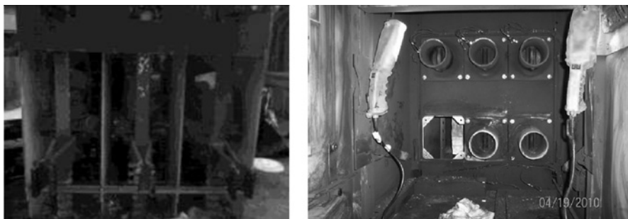
Figure 19.6 Aftermath of an arc flash in a 13.8 kV breaker.
