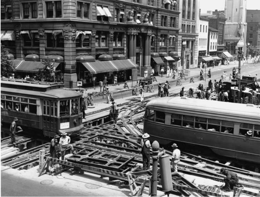
Figure 2.3: Seen here in the 1940s is the intersection of 14th and G Streets NW in Washington, D.C., where two lines crossed and there was a set of connecting tracks. Laborers are making repairs both above and below the surface. While the design of the electric conduit system is not fully evident in this view, what is visible suggests an astonishing complexity. Note, however, that there is not one wire to be seen anywhere above ground. (Capital Transit Company photo, author's collection)
