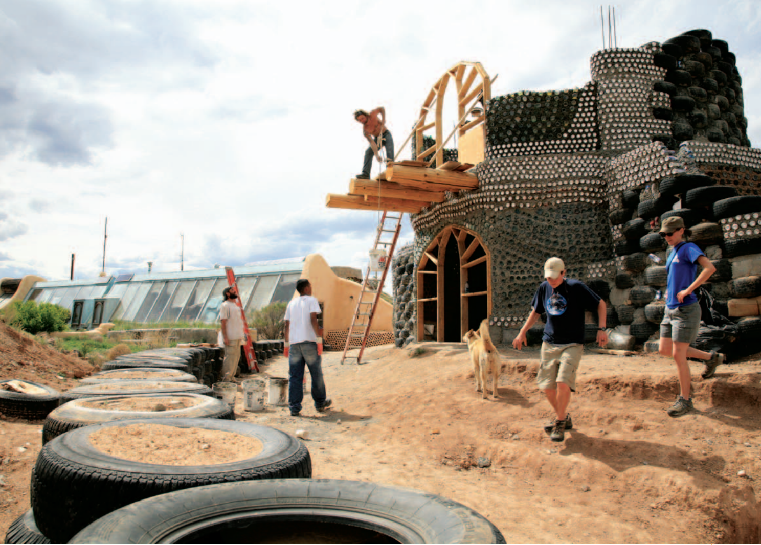
Builders use tires, bottles, cans, and plain old dirt to make Earthships.
