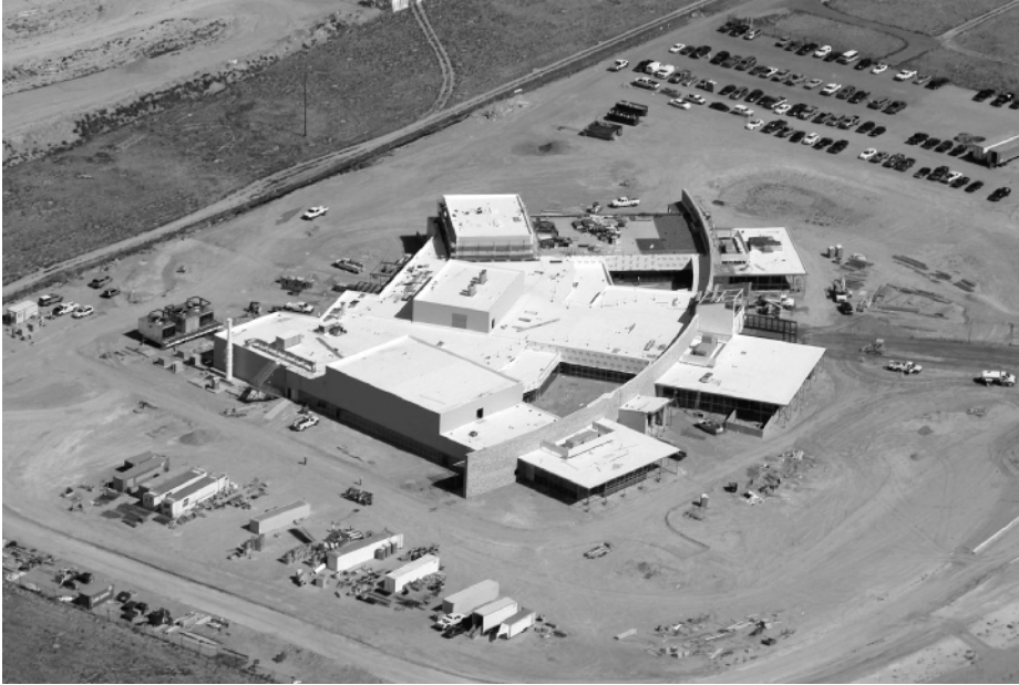
Figure 1-6 This is an aerial view (taken in September 2005) of the hub facility of the new Sandia/Los Alamos joint Center for Integrated Nanotechnologies (CINT) in Albuquerque, New Mexico. The building's three wings house a characterization lab (containing the most vibration sensitive instruments), a synthesis lab (which includes physical, chemical, and biological facilities), and clean room facilities for device integration activities at the nano/microscale level. (Credit: Photograph courtesy of U.S. Department of Energy/SNLA.)
