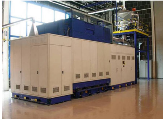
Fig. 5.95 The CHP 100 SOFC generator by Siemens at turbocare in Turin
