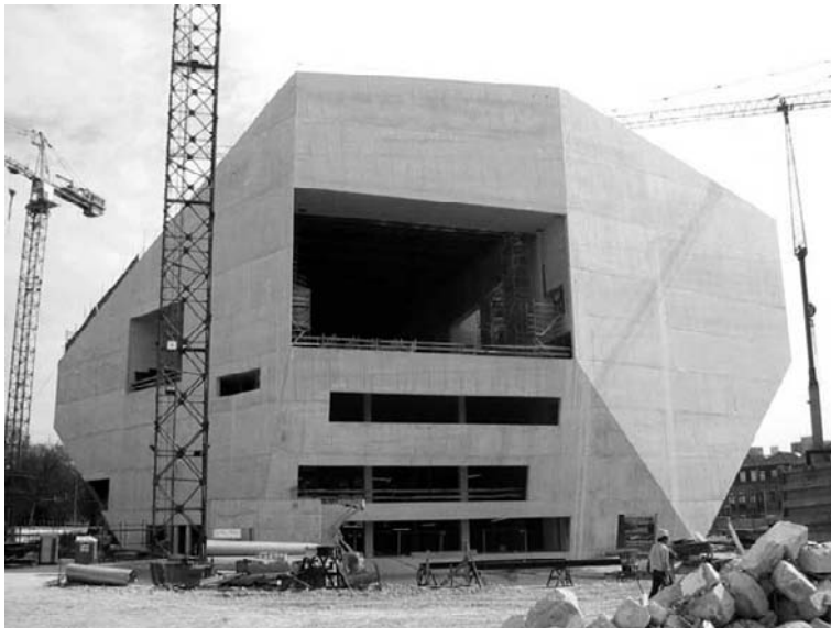
Fig. 3. The white concrete shape of the Casa da Musica during construction. Notice the large window in front.
