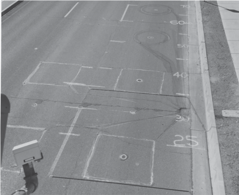
Figure 8.23 Oracle Road showing surface and subsurface sensors and paint for calibrating the VDS field of view. The inductive loops and magnetometers at the center of the loops have also been outlined.
