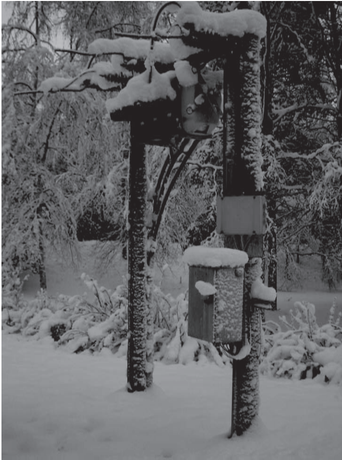
FIGURE 4.14 Overhead customer substation showing transformer and, at the pole top, an ice-encrusted air break switch.
