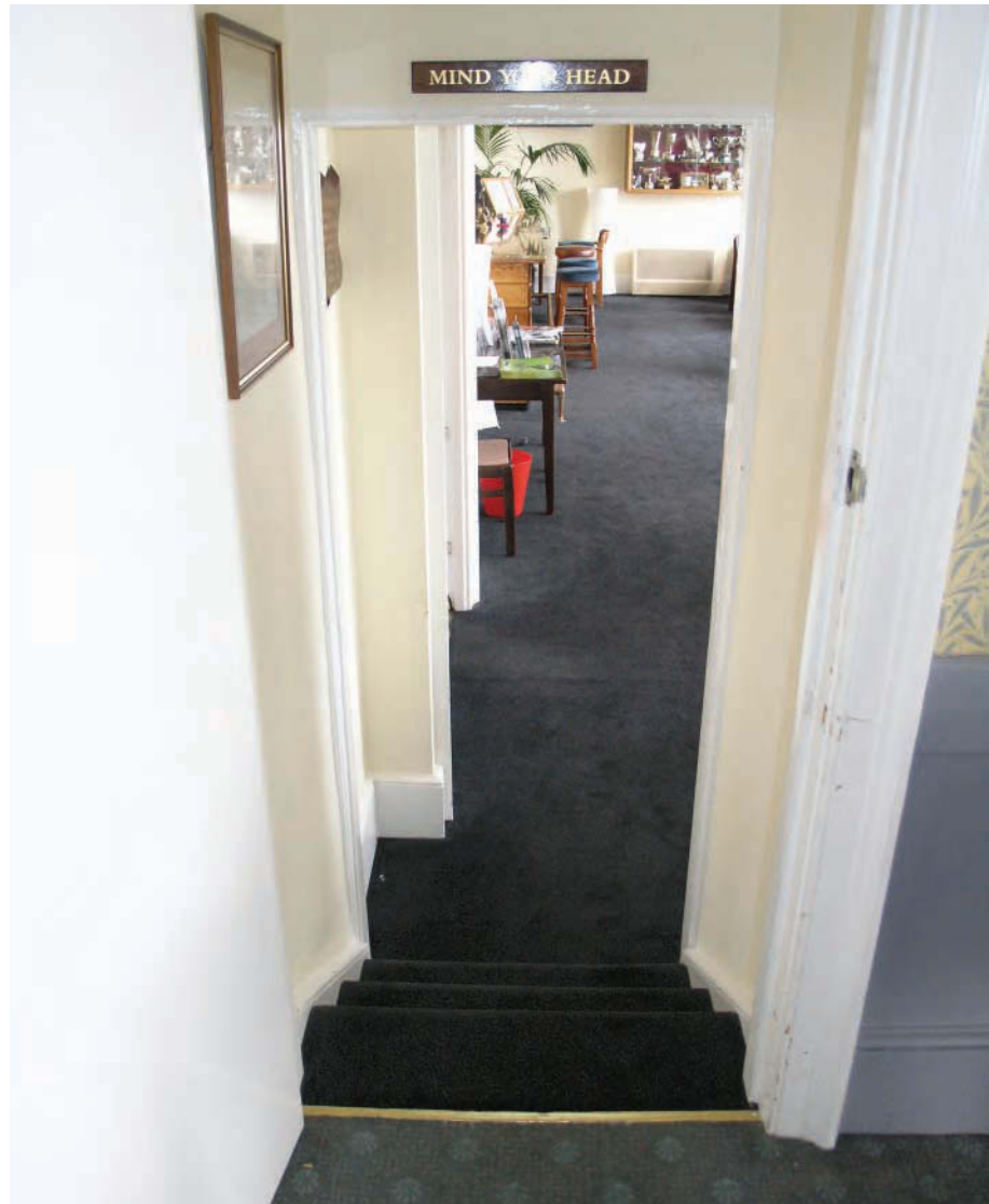
Plate 16 A typical stair hazard; it is difficult to discern the edges of the treads
