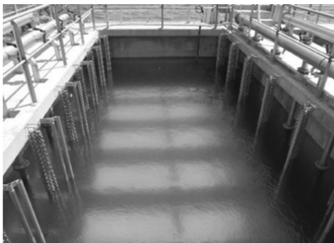
Figure 2.5 Upgrade with MBR of the wastewater treatment plant of Aigio city, Greece for 30,000PE.
