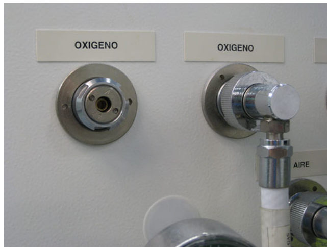
Figure 13.4. Three-tooth wall outlet specifically for oxygen in the operating room. Note the air connector below and to the right of the oxygen connections.
