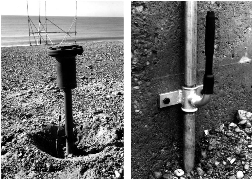
Stand alone monitor system (left) — sensors mounted on stem with data logger in head unit and (right) single scour sensor (photographs courtesy of HR Wallingford)
