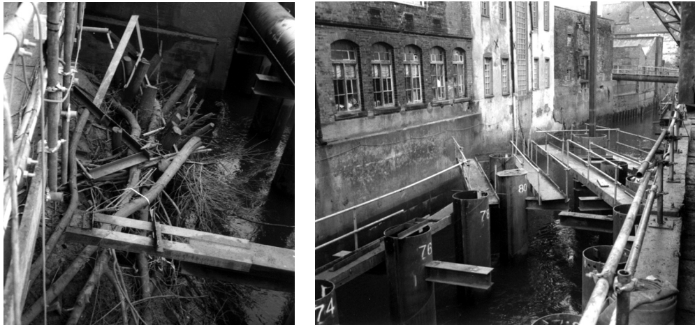
Piling close to waterfront buildings was delayed by the need to remove tree stumps that had been cut off near bed level (photographs courtesy of S. Kent, Environment Agency)
