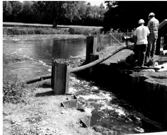
Outflow from diversion channel into downstream channel
