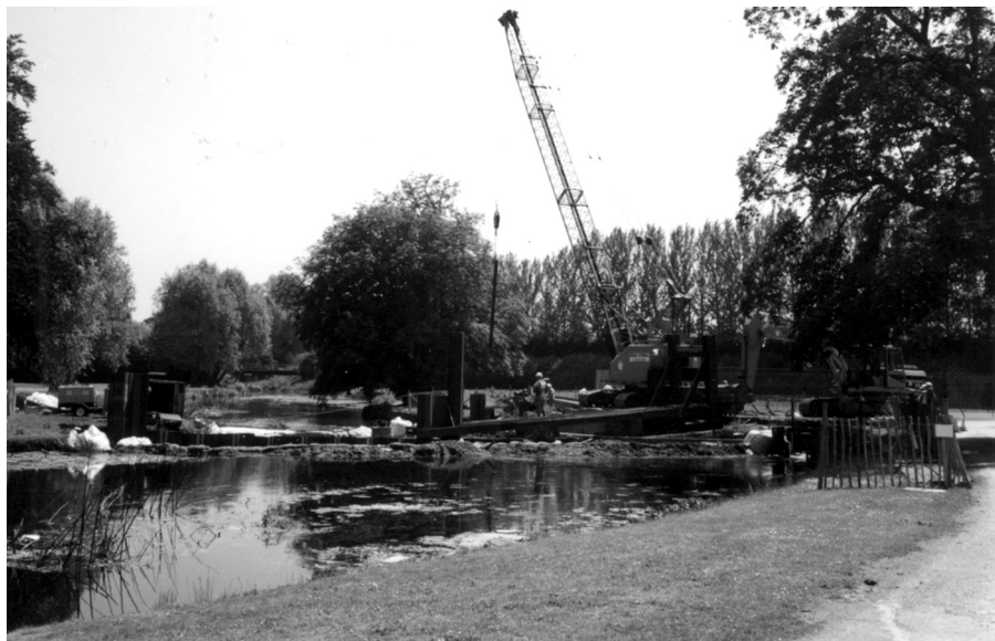
View from upstream. River diverted by a temporary earth bund into the diversion channel on the right-hand side. Access for crane via the temporary bridge over the channel
