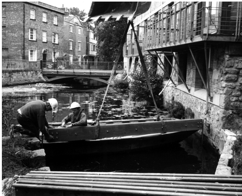
Trash boom being installed at a new weir (photographs courtesy of HR Wallingford)
