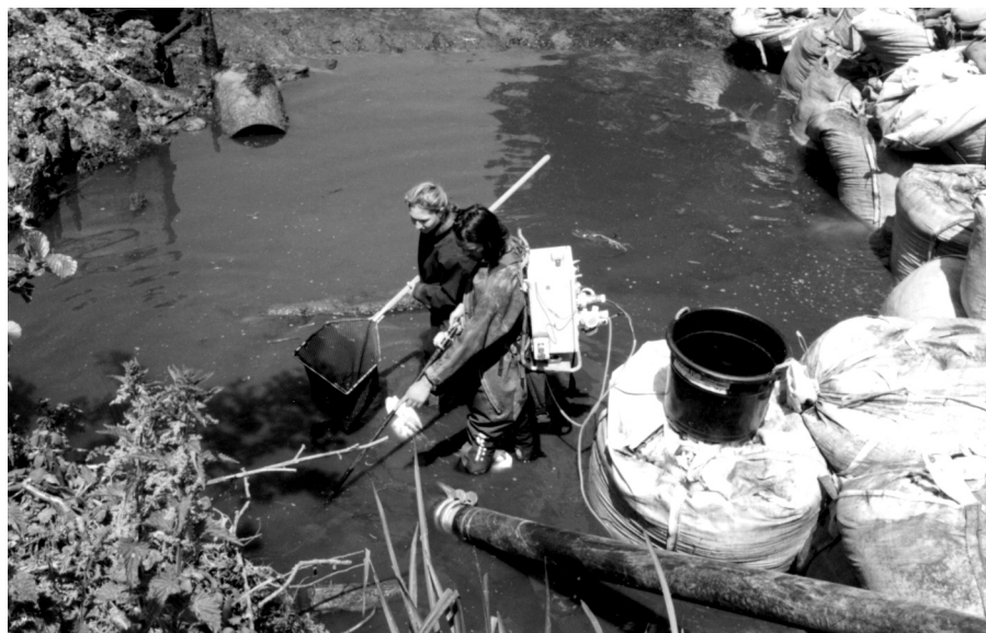
Following successful bunding of the old weir, fish were removed from the enclosed pond and released into the river downstream (Photographs courtesy of HR Wallingford/Environment Agency)
