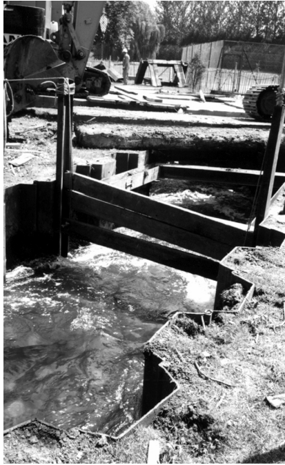
Inlet to diversion channel — flow controlled by boards as required
