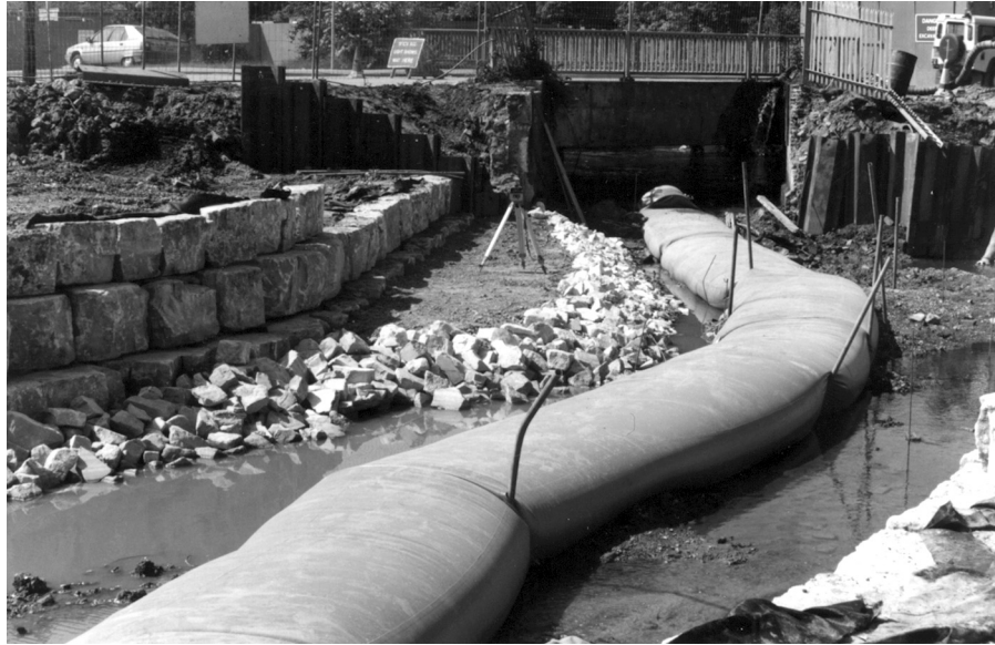
Downstream discharge point for pipework (note environmental stonework features to enhance habitat) (Photographs courtesy of HR Wallingford/Environment Agency)
