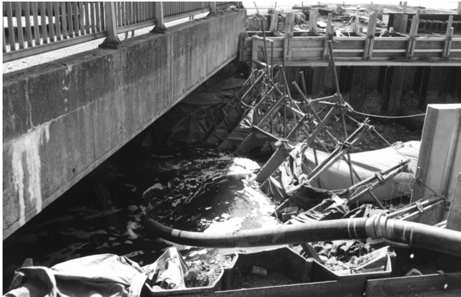
PortaDam with entrance to pipe running through the site
