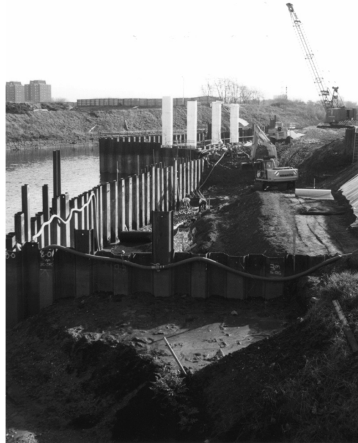
Looking downstream along right bank (photographs courtesy of HR Wallingford/Sir Robert McAlpine)
