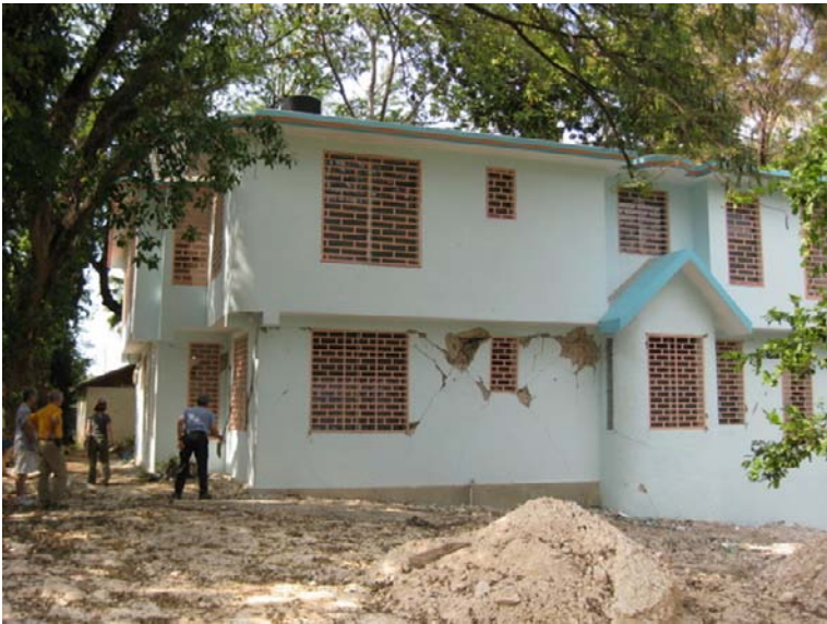
Figure 2: Newly constructed building which is a hybrid of reinforced concrete and CMU block.
