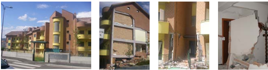
Figure 8: The dwelling building of Via Borgo dei Tigli 6-8-10 in L’Aquila (Pianola area), just completed before the 2009 Abruzzo earthquake (left) and damage caused to the building by this event. Its retrofit by means of HDRBs and SDs has been planned, with safety certification of A. Martelli.
