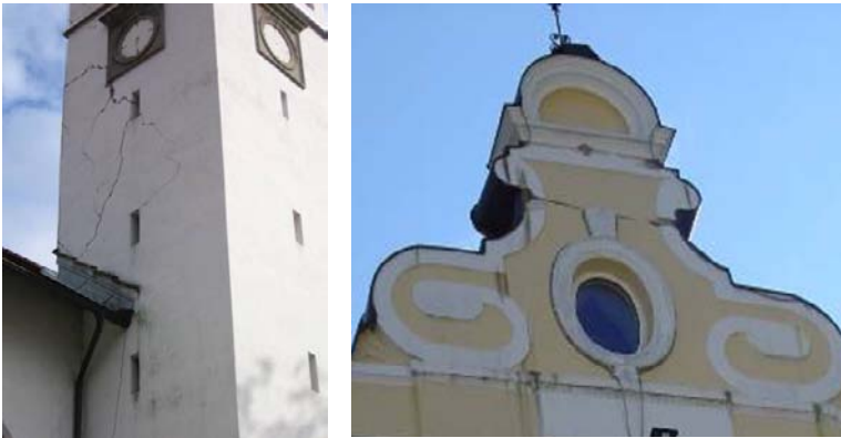
Figure 2: Typical damage on bell tower of a church and console structure of a historical building.
