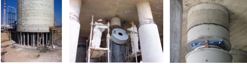
Figure 5: One of the three tanks of the company Polimeri Europa of the Italian ENI Group located in Priolo Gargallo (Augusta, Syracuse, seismic zone 2*), which were seismically retrofitted using U.S. FPS devices in the years 2005-2008 and one of the isolators during and after its installation [4] (this is the only application of SI to chemical plants and components so far existing in Italy; prior to the 2009 Abruzzo quake, it was also the only Italian application of CSSs).
