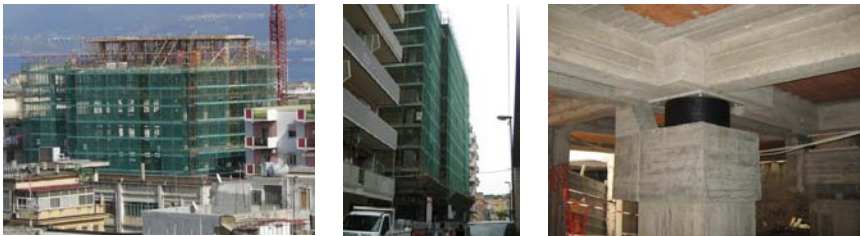
Figure 4: A new 8-storey dwelling building being erected in Messina, in seismic zone 1 (June 2010), the tallest isolated Italian building (its safety will be certified by A. Martelli), and one of the LRBs forming its SI system together with SDs.
