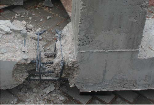
Figure 9: Photograph of the ultimate rupture of prototype 5.
