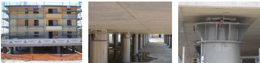
Figure 6: One of the 184 pre-fabricated houses (wood, or r.c., or steel structure) erected in l’Aquila for homeless residents after the 2009 Abruzzo earthquake and some of the 40 CSS devices, manufactured in Italy, installed at the top of columns to isolate its supporting slab (the lower floor is used as garage).
