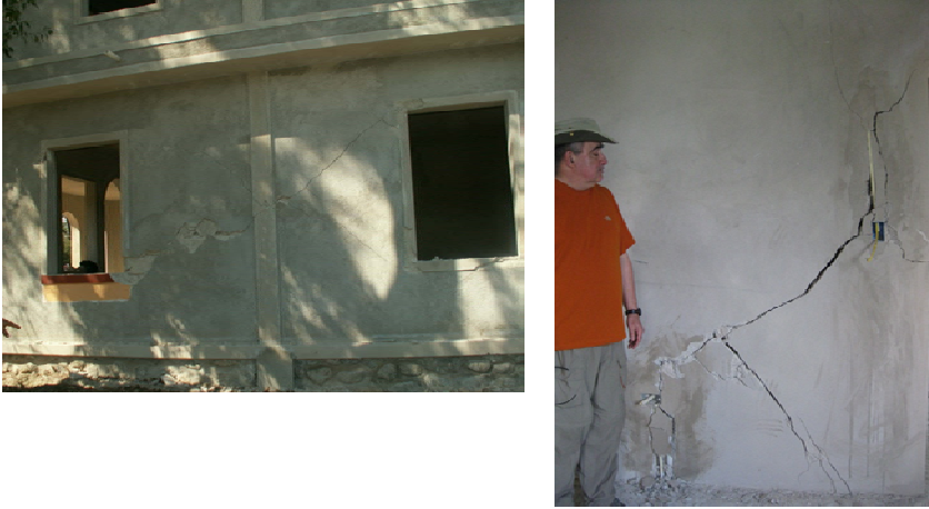
Figure 3: Wall shear failure in newly constructed hybrid reinforced concrete and CMU block (left outside view, right inside view).
