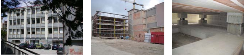
Figure 7: The Romita High School for scientific studies (1,300 students) in Campobasso (seismic zone 2) prior to the demolition of its blocks “A” and “B” (left); reconstruction of block “B” in progress in October 2010 (at the centre); two HDRBs and one SD in its underground technical floor (right).
