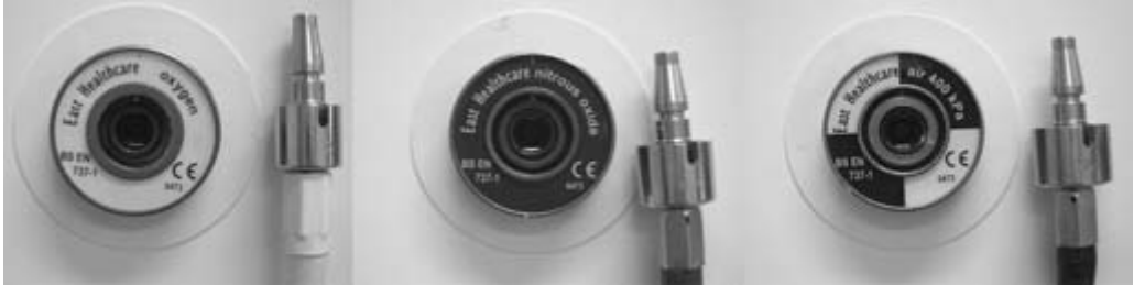
Figure 2.11 Wall-mounted outlets and gas-specific probes for (left to right) oxygen, nitrous oxide, air.
