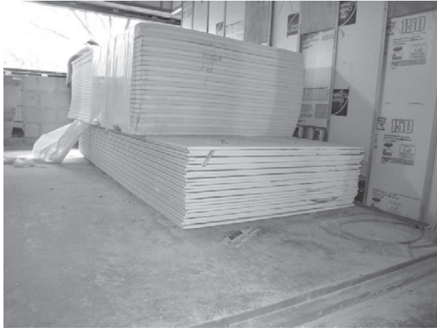
Insulation ready to be installed, kept off the ground
