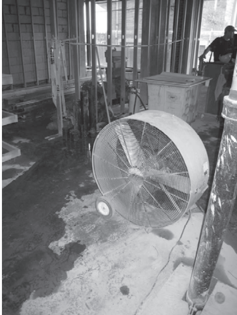
Temporary ventilation fan used during construction
