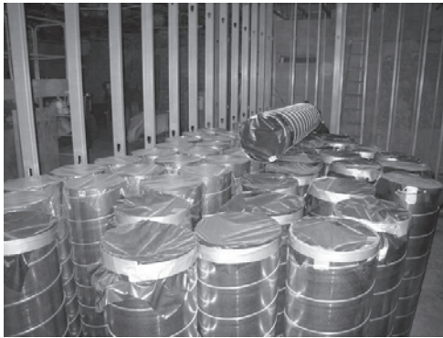
Ssealed Ducts – before installation
