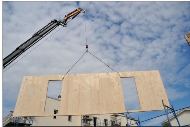
An example of building a panelized home. Note the section of a home being raised so that it can be assembled with additional prefabricated walls. As you can imagine, homes can be built more quickly using this innovative method of construction.
