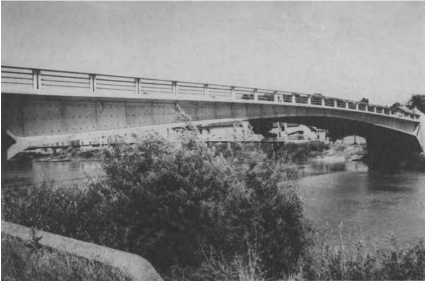
Fig. 16-17. The Esbly bridge over the Marne River in France. (Provided by and reproduced with the permission of the Freyssinet Company, Inc., Charlotte, N.C.)
