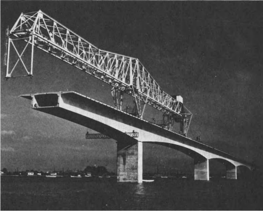
Fig. 16-18. The Oléron Bridge in France. (Provided by and reproduced with the permission of the Freyssinet Company, Inc., Charlotte, N.C.)
