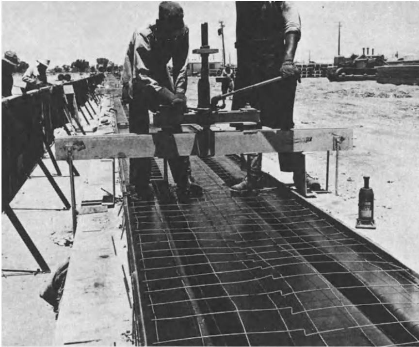
Fig. 15-15. Hold-down device shown spanning a double-tee form with workmen in the process of deflecting the tendons with a hydraulic jack. (Provided by and used with the permission of the FMC Corp., Chicago, Illinois.)
