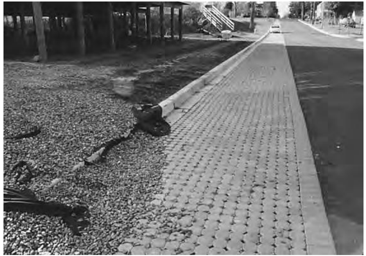
Figure 32. Unwanted sediment tracked onto permeable pavers via this gravel access ramp to a construction site will clog their openings.
