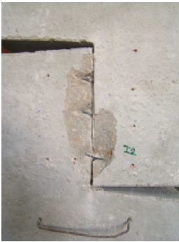
Precracked SCC with TR
