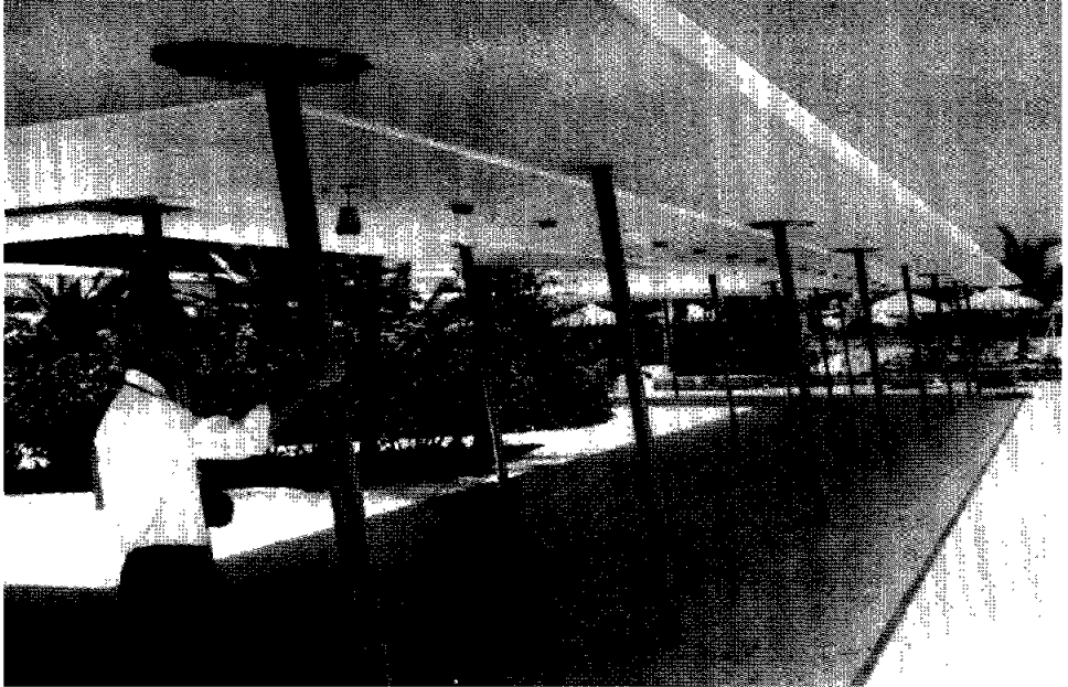
Figure 1.1.1 This pergola at the Macuto-Sheraton Hotel near Caracas, Venezuela was damaged by the earthquake of July 29, 1967. The Magnitude 6.5 event, which was centered about 15 miles from the hotel, overstrained the steel pipe columns. (Courtesy of G. W. Housner.)
