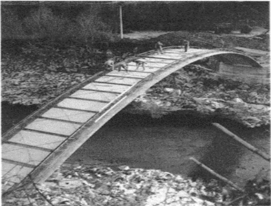
Figure 10 Soča Bridge after placements of whole concrete slabs and the first concrete between them
