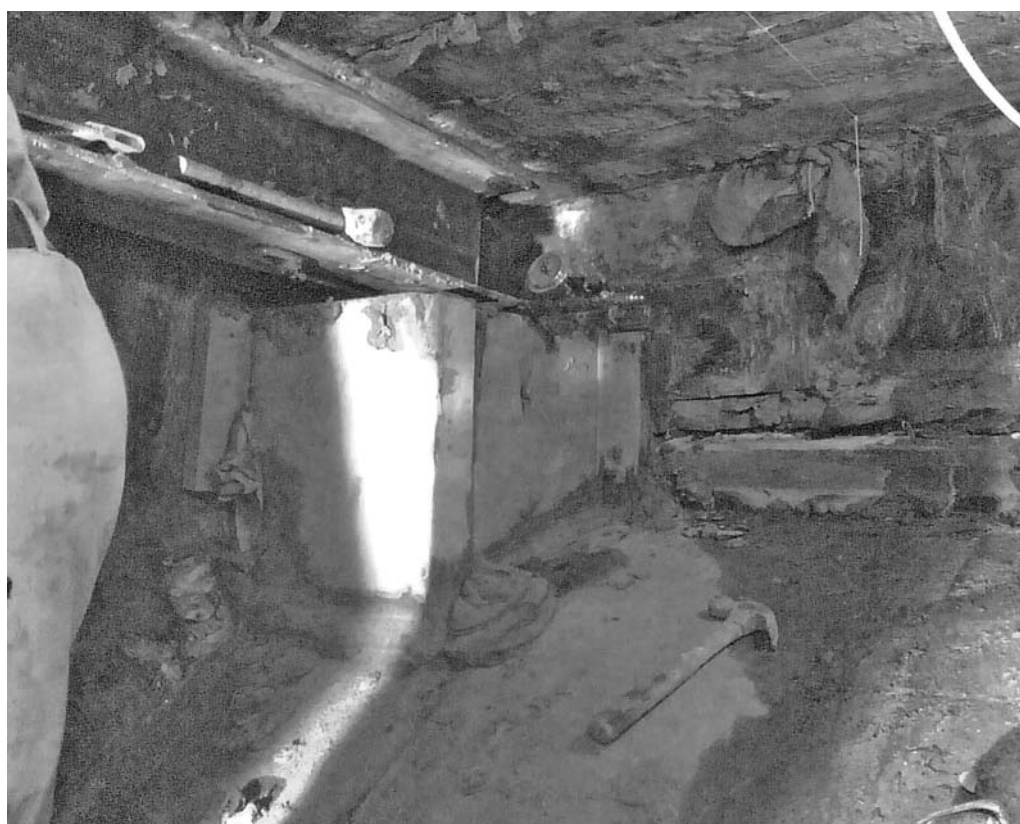
Figure E.4. Typical example of where monitoring could be used in a heading
