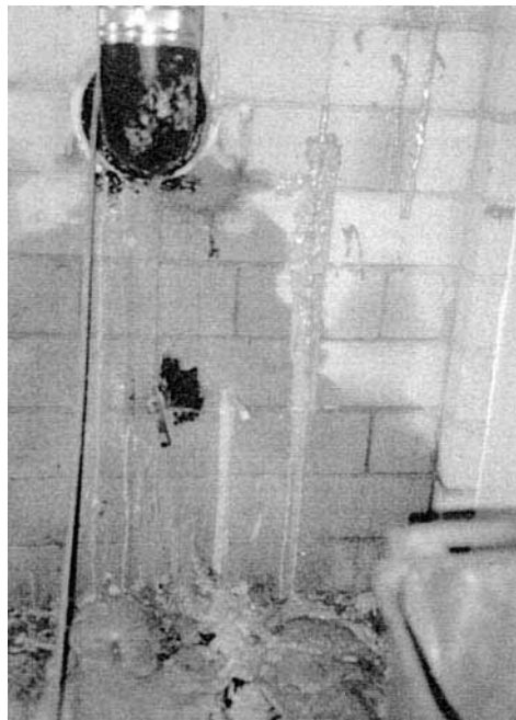
FIGURE 6B.114 Reacted grout on wall.
