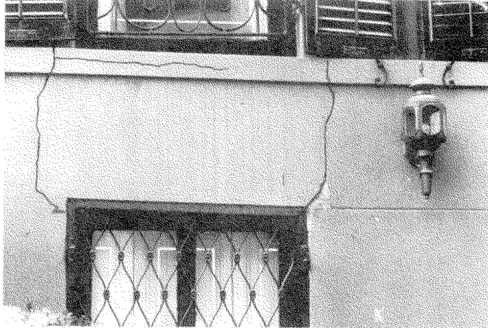
FIGURE 7.5 Structural damage caused by adjacent excavation.
