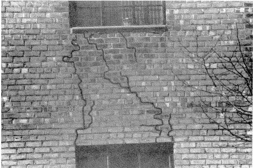
FIGURE 8.37 Masonry cracks due to settlement.
