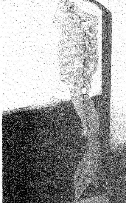
FIGURE 8.72 Interior distress (see Figure 8.71).
