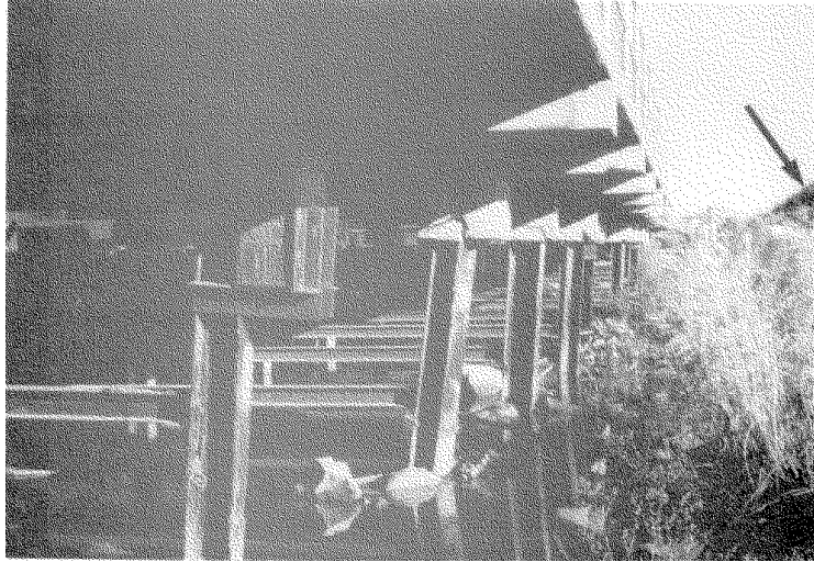
FIGURE 8.27 Lateral soil shift causes pile failure.
