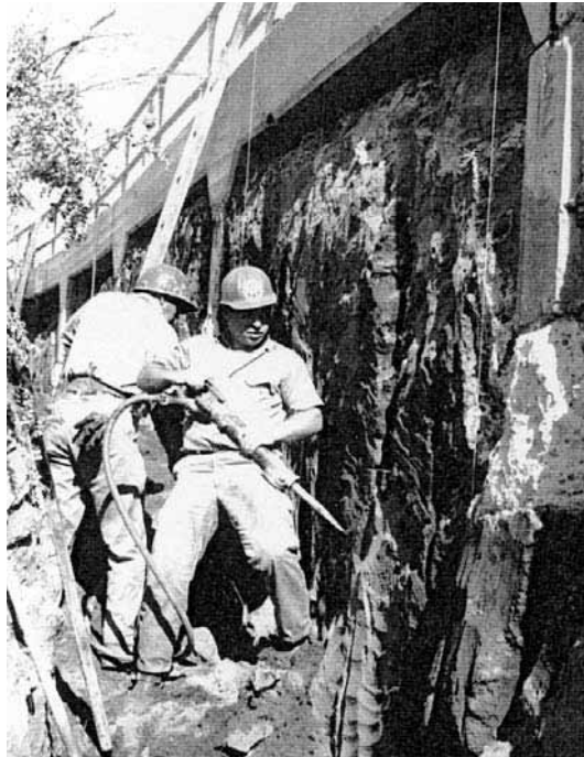
FIGURE 6B.98 Solidified mass allowed excavation of shear vertical cut, including removal of part of the supporting concrete footings.
