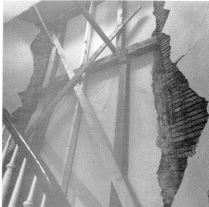
FIGURE 8.19 Cracking of partition wall and settlement of stairs due to footing movement.
