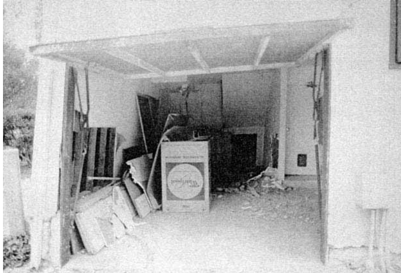
FIGURE 6B.52 Structural distortion caused by blow out of a retaining wall.
