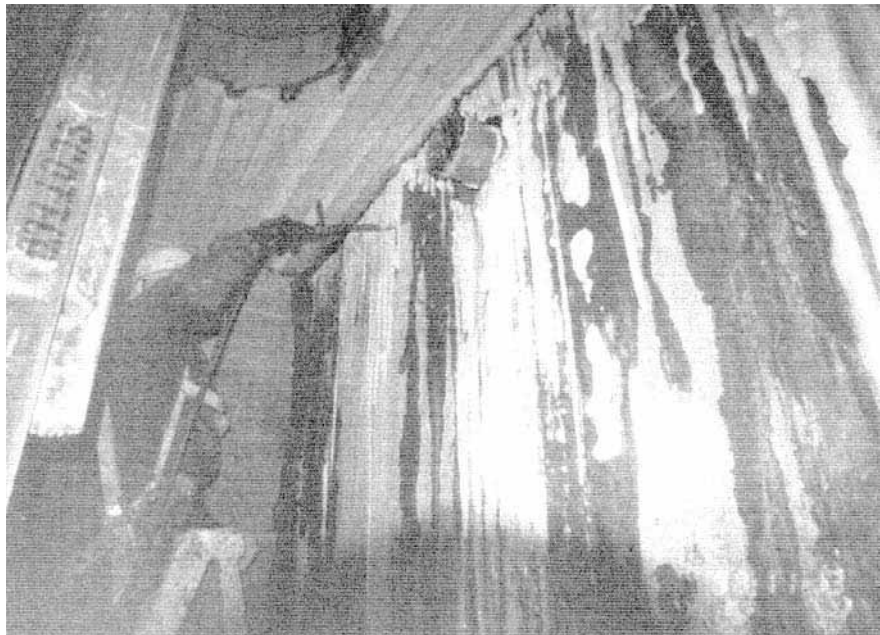
FIGURE 6B.13 Hydrophilic urethane grout spills are extremely difficult to clean up.
