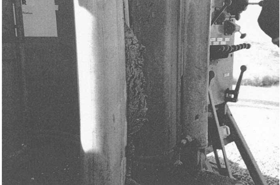
FIGURE 6B.55 Grout escaping from split casing.
