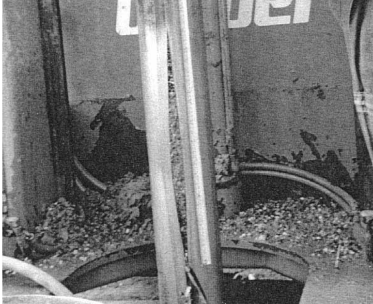
FIGURE 6B.140 Split of casing that resulted in sudden drop of injection pressure.
