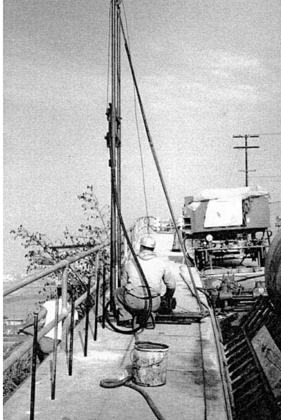
FIGURE 6B.99 Special needles were driven to the depth of injection, which proceeded from the bottom, up.
