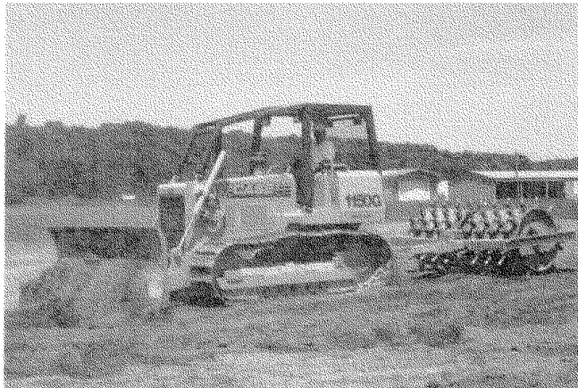
FIGURE 6A.17 Tracked bulldozer towing a sheepfoot roller (courtesy of Case Corporation, Racine, WI).
