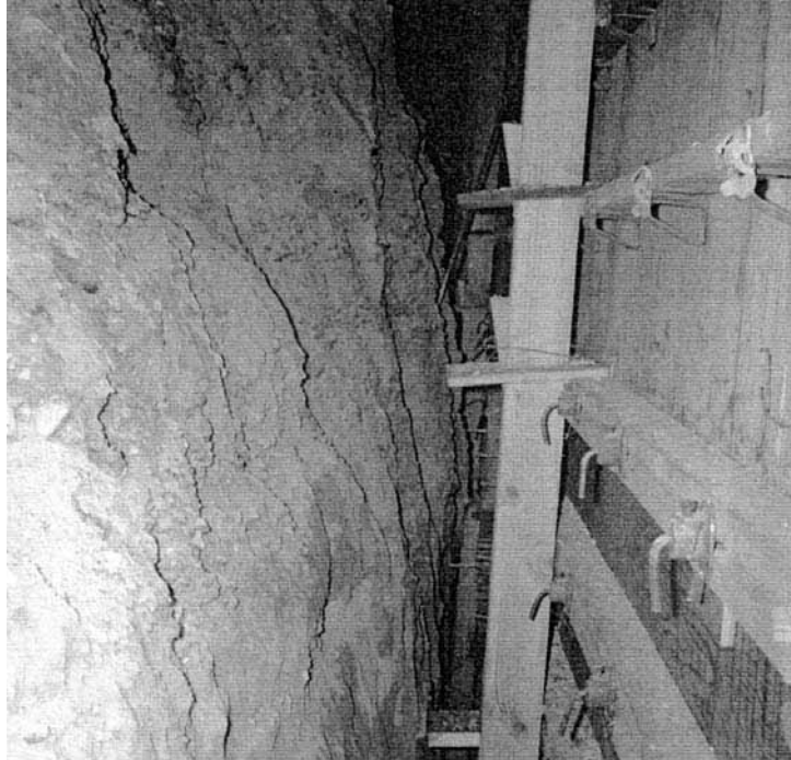
FIGURE 6B.102 Formwork for the new foundation, adjacent to near vertical cut of cohesionless soil.
