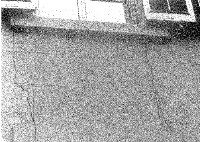
FIGURE 8.18 Damage resulting from excavation.
