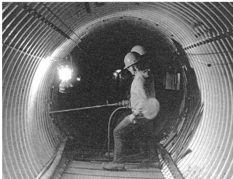
FIGURE 6B.77 Drilling of 12 foot long radial grout holes from inside drainage conduit.
