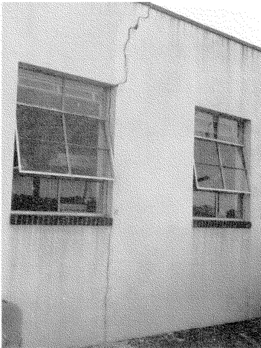
FIGURE 8.69 Masonry distress caused by soil shrinkage (loss of bearing support).
