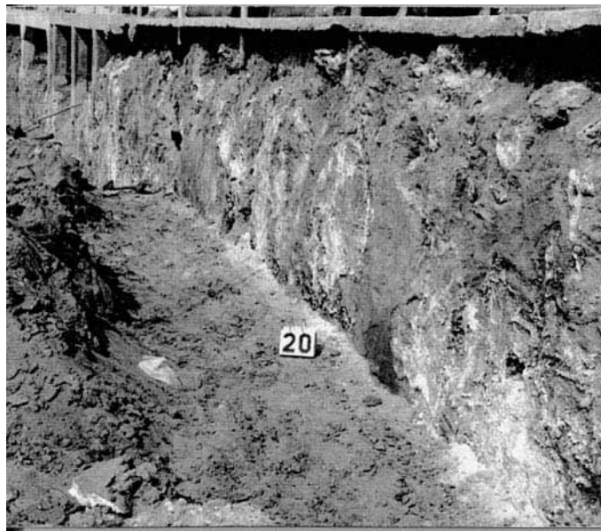
FIGURE 6B.11 Cohesionless dune sand solidified with a chemical solution grout enable support of vertical excavation.
