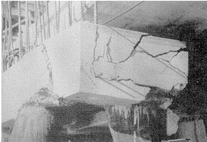
FIGURE 8.48 Failure of concrete pile caps due to ice action.
