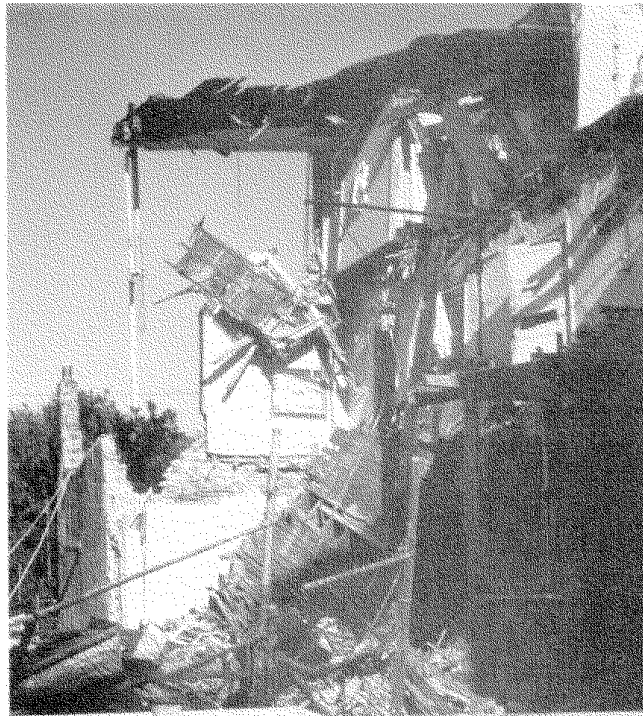
FIGURE 8.9 Building collapse—ineffective bracing.
