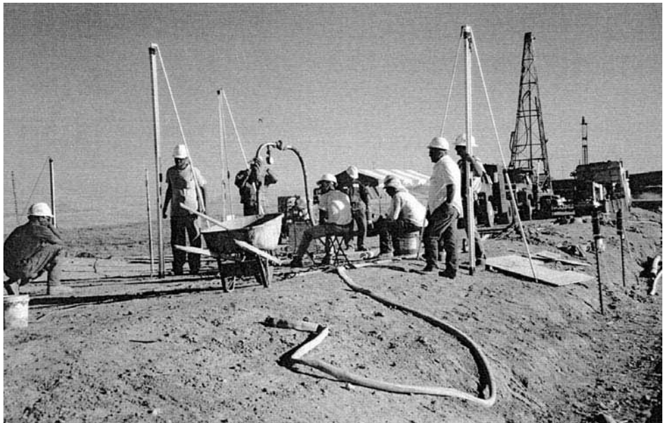
FIGURE 6B.86 Remedial grouting in progress. Note survey activity to ensure against any surface heave or other movement.
