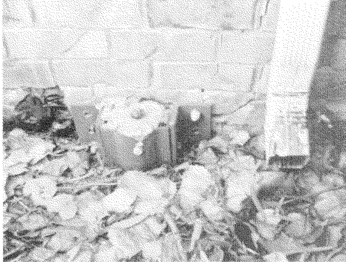
FIGURE 7B.4.10. This photograph illustrates one of the problems that can occur as a result of using the perimeter beam as the resistance to drive a steel minipile. Not only have the bolts sheared (losing all support for the structure), but the foundation beam has also been seriously sheared.
