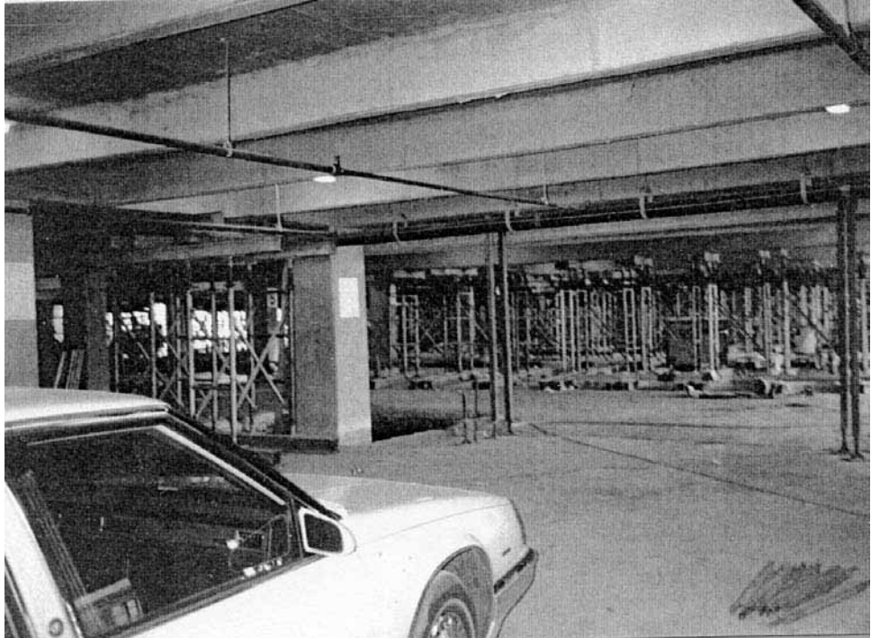
FIGURE 6B.131 Groutjacking was used to precisely level pile-supported columns of parking structure.
