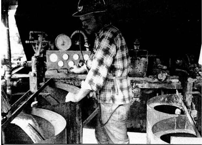
FIGURE 6B.109 Grout mixing and pumping plant.
