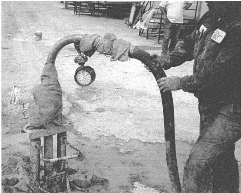
FIGURE 6B.36 Typical connection to a grout hole during upstage injection. Note pair of hydraulic jacks used for casing extraction.
