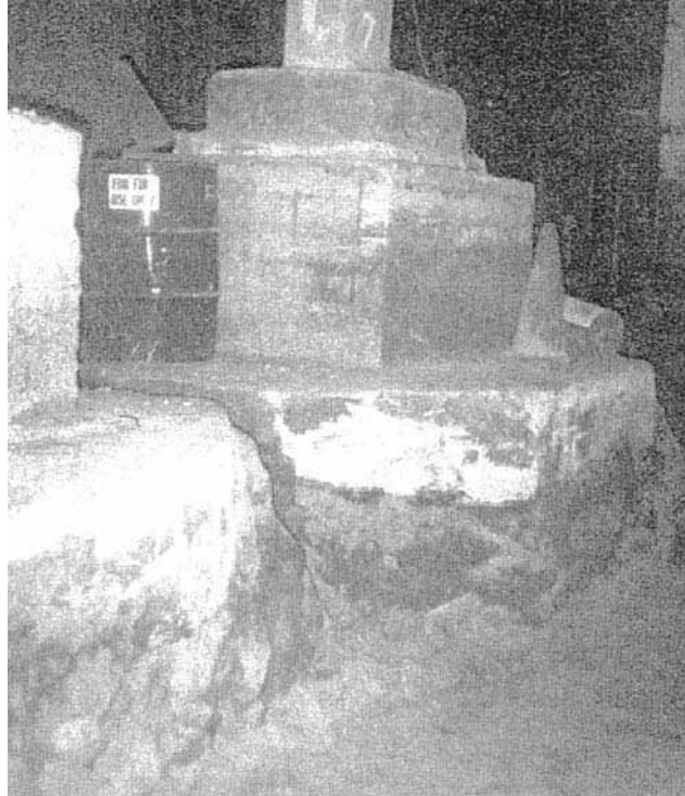
FIGURE 6B.90 Ultrafine cement grout used to solidify cohesionless sand allows excavation under the foundations of a structure.
