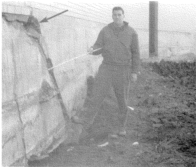
FIGURE 8.65 Foundation wall failure during construction.
