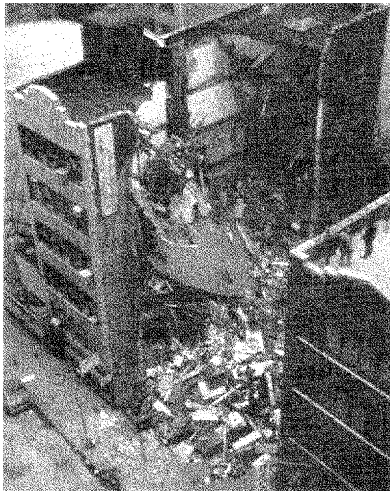
FIGURE 7.6 Building collapse caused by adjacent excavation.
