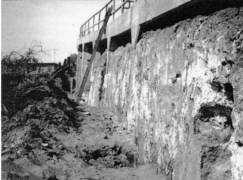
FIGURE 6B.100 Vertical cut face varied from 6 feet to 24 feet high and extended for 240 feet.
