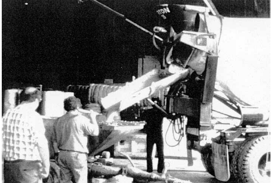
FIGURE 6B.128 Fill grouting of large voids with ready-mixed mortar and a standard concrete pump.
