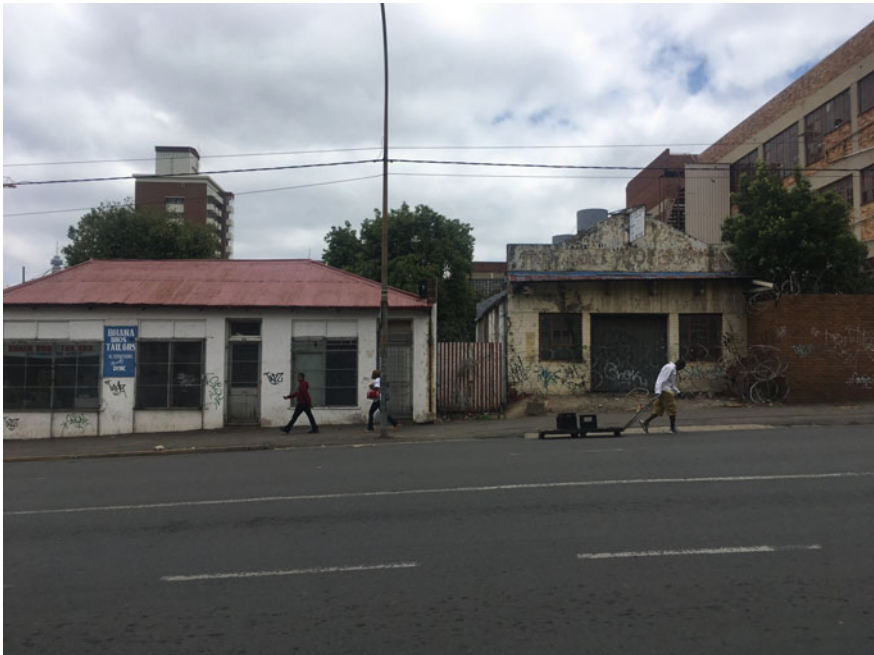
Fig. 5.3 Buildings in ruin and neglect opposite the Maboneng Precinct. Image by the author
