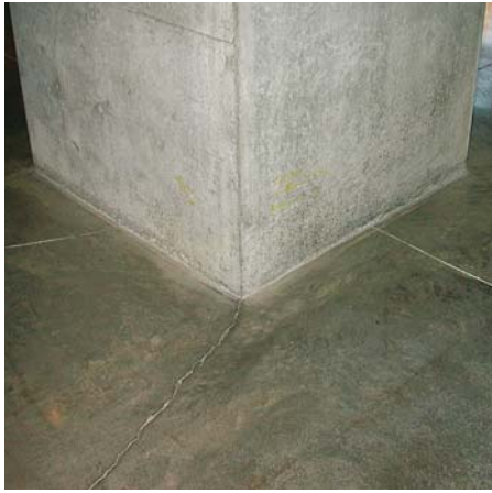
Cracks in the floor slab around an interior column oppose the anticipated crack direction. Cracking can be caused by improper isolation-joint design that does not provide relief at reentrant corners.
