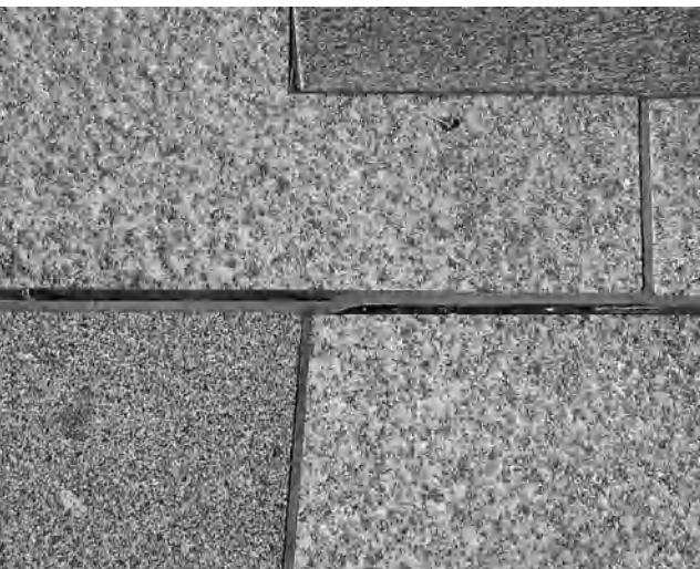
Adhesion failure of sealant on stone.
