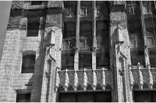
Terra-cotta blocks netted over to prevent from falling to the streets, Mather Tower, Chicago, 1928.
