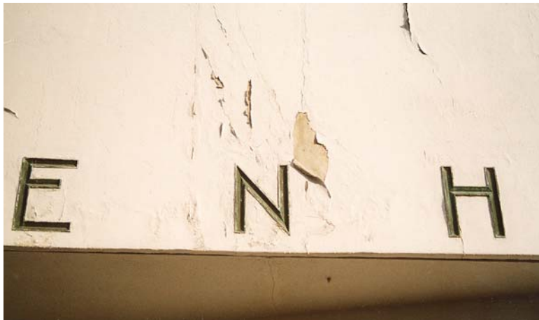
Guggenheim Museum, New York. The façade is frequently in disrepair and needs to be painted every four years.
