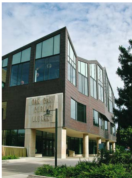
below Staining of concrete walkway was an inevitable consequence of installing copper cladding on Oak Park Public Library, Chicago completed in 2003 and designed by Nagle Hartray and Associates.
