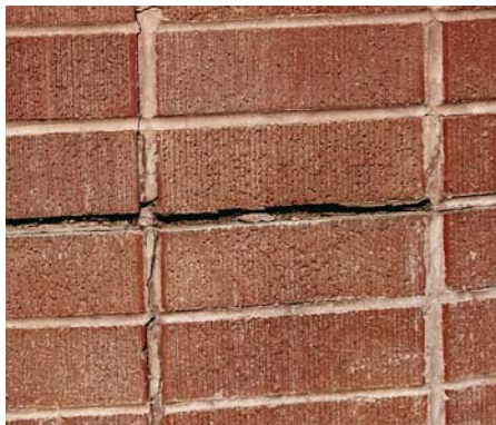
right Corrosion of masonry joint. Giraffe House, Denver Zoo.
