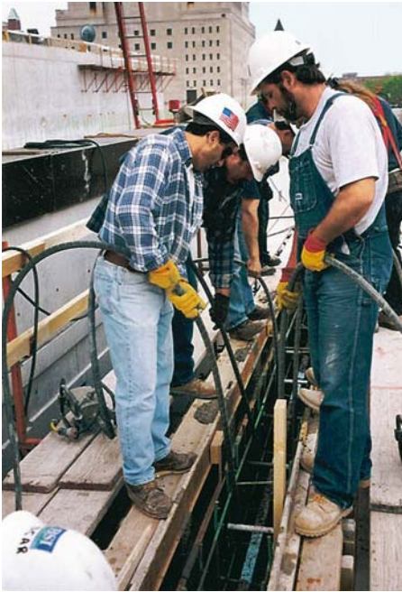
Extensive vibration is required during pours to remove air pockets that can lead to surface defects. Pulitzer Foundation, St. Louis.
