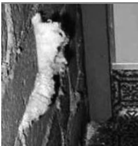
Crystallized efflorescence in a masonry wall.
