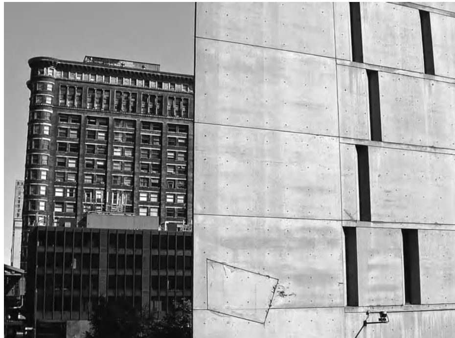
below Dripping water from an air-conditioning unit is the cause of efflorescence on this masonry wall.
