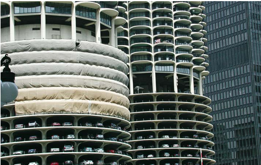
Open concrete balconies are susceptible to reinforcement corrosion caused by weather and de-icing salts. Marina Towers, Chicago.
