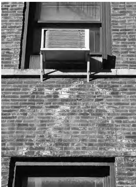
right Spalled concrete at window detail. Metropolitan Correctional Center.
