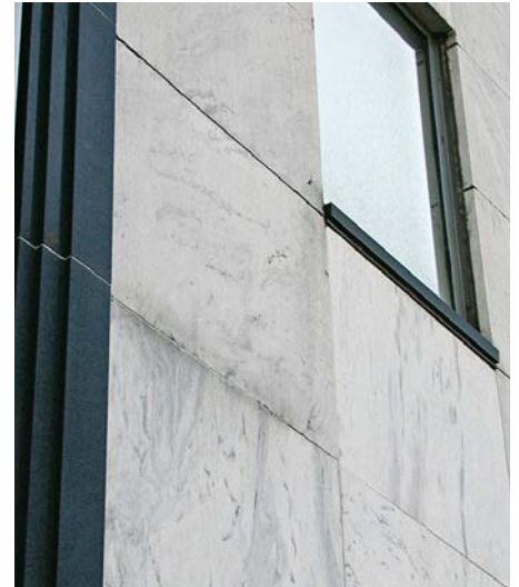
Silicone sealant can stain white marble.
