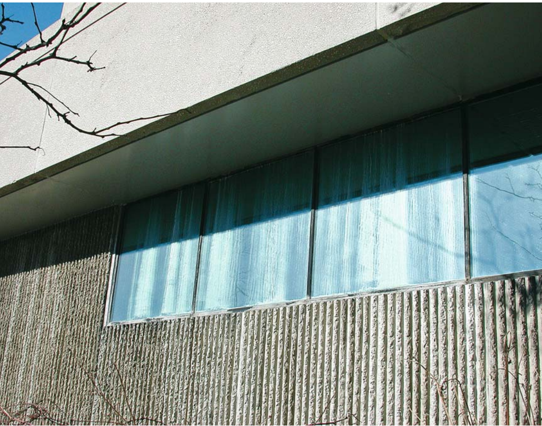
right Image of white corrosion marks on glass from concrete runoff.
