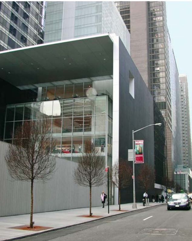
The MOMA expansion in New York City brought large concentrated loads on the garden pavers. The result was broken paving blocks.
