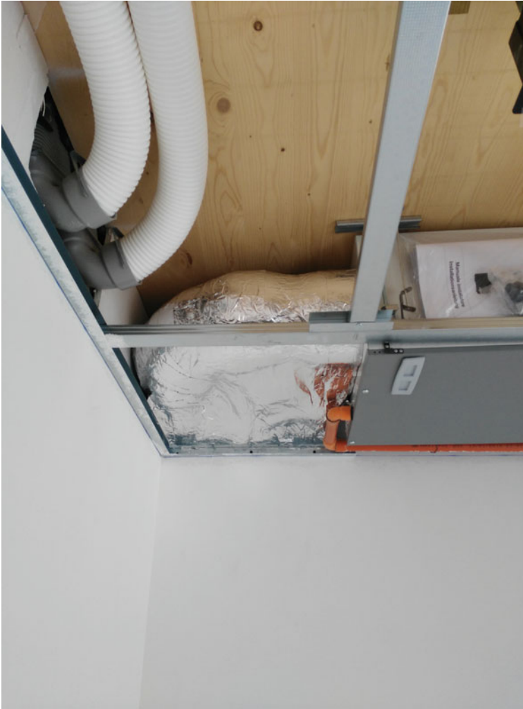
Fig. 9.7 Detail of the previous image after further insulating material has been introduced in the tubes of extracted and consumed air
