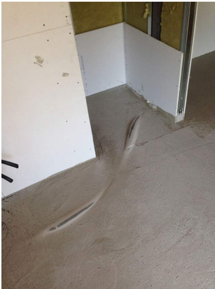
Fig. 9.18 Ventilation duct that emerges from the lightened screed. To allow good airtightness of the 5-cm-thick cement screed, it is necessary that the pipes do not protrude from the lightened screed by more than 1 cm
