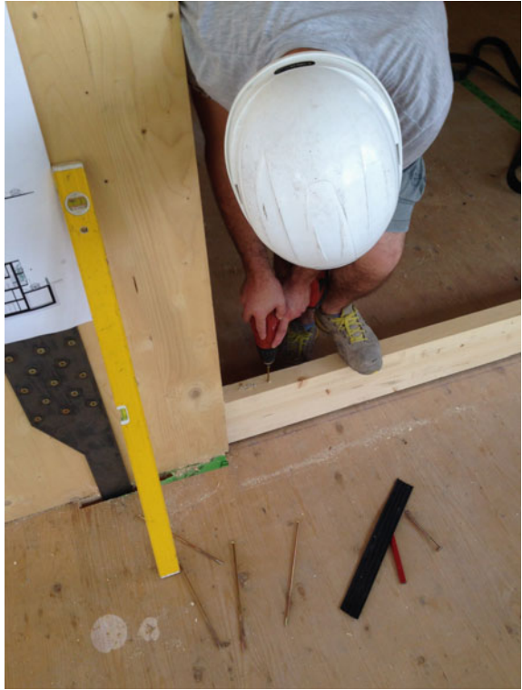
Fig. 4.32 Laying of the strip in larch wood in order to ensure the application of the waterproofing and the subsequent installation of the French doors
