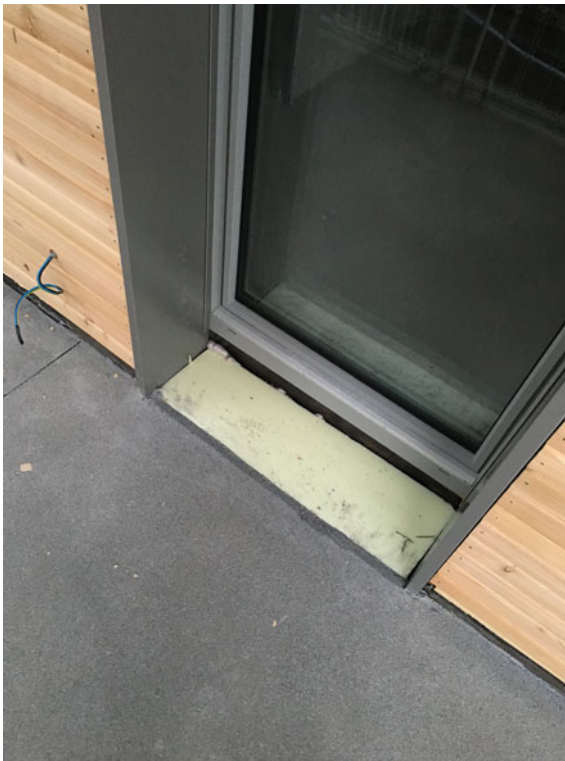
Fig. 7.40 Lower installation of the French door after the pouring of the cement screed on the terrace
