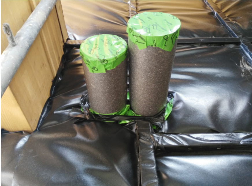
Fig. 8.14 Sealing tape applied on the output channels of the controlled mechanical ventilation system (internal side)
