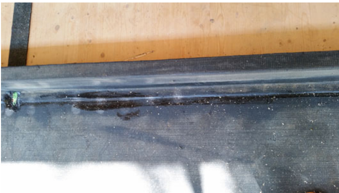
Fig. 4.33 Application of waterproofing sheath on the terraces and on the strip in larch wood used for the anchorage of the French doors
