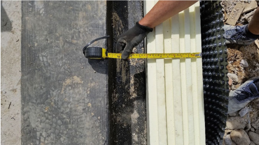
Fig. 4.23 Detail of the panels in the XPS used for insulating the foundation kerb
