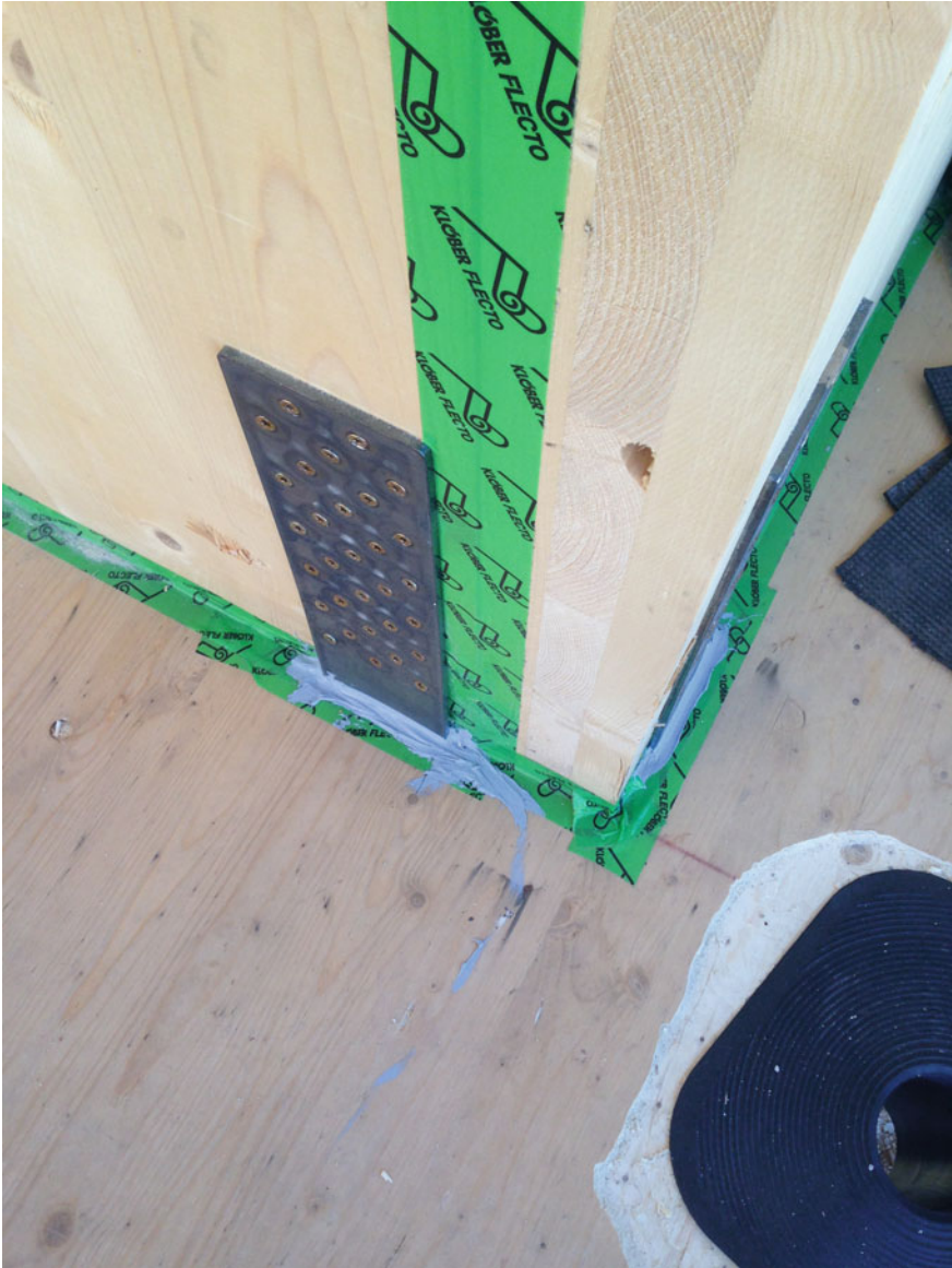
Fig. 8.4 Sealing of the joints on the external side with sealing tape and silicone sealing on the anchorage plate
