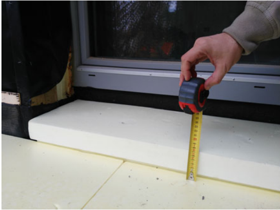
Fig. 7.39 Lower installation of the French door where insulation in XPS was installed for the protection of the thermal bridge of the stone threshold
