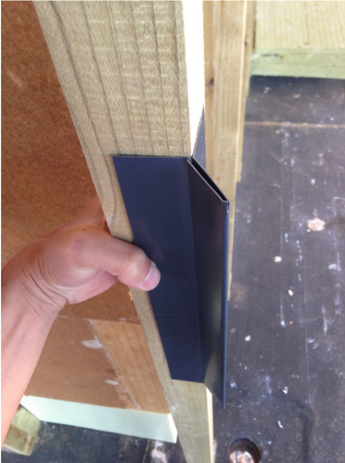
Fig. 7.27 Solution of the corner with the profile in aluminium sheet that accommodates the planks of larch wood with head cut at 45°
