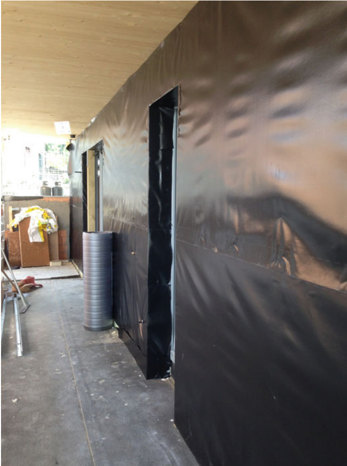
Fig. 5.8 Wind barrier membrane (incorrect installation)
