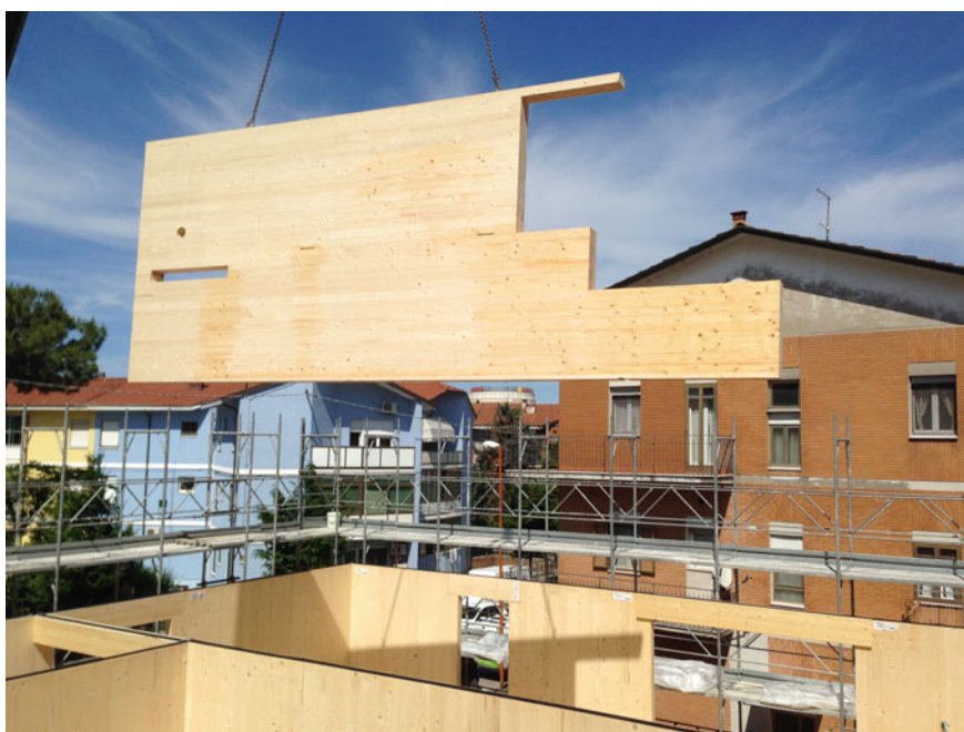
Fig. 4.11 Lifting a panel in CLT that has been shaped in the production plant
