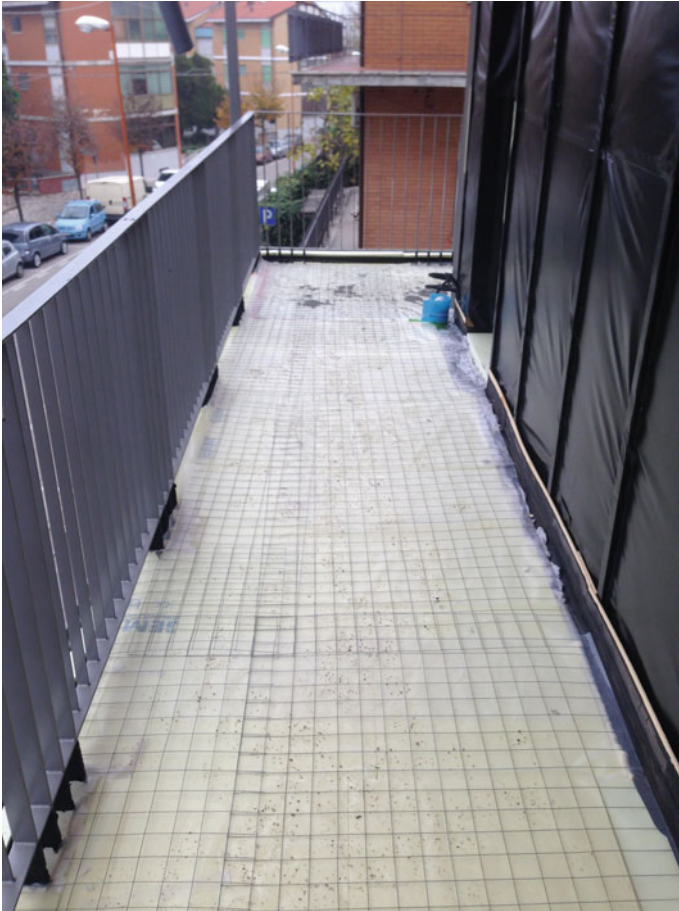
Fig. 7.16 XPS panel ready to receive the laying of the cement screed in which a metal mesh is inserted
