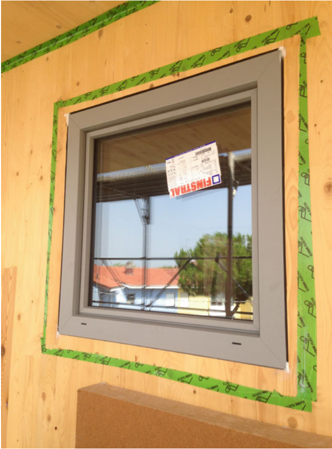
Fig. 7.35 Installation of the window directly in the panel in CLT without the use of the subframe
