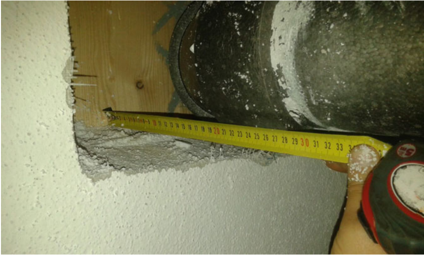
Fig. 5.20 Inspection hole on the wall clad in EIFS to check the thickness of the panel in EPS
