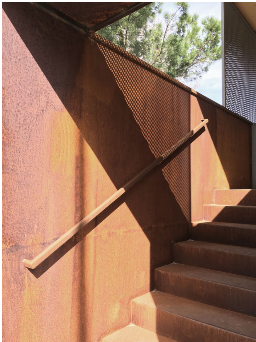
Fig. 11.26 Detail of one of the accesses on Via Liguria made in Corten steel sheet
