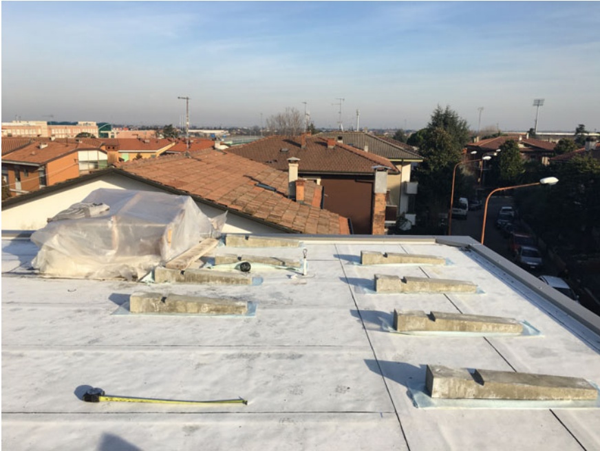
Fig. 7.22 Processing of the finished roof, highlighted are the weights in cement for the laying of the photovoltaic panels
