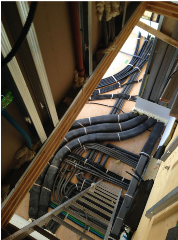
Fig. 9.16 Distribution of the technical systems in an apartment seen from the stairwell
