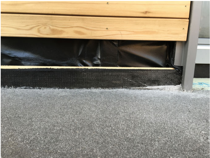
Fig. 5.10 Waterproofing in the point of contact of the wall with the terrace. The waterproofing sheath will be covered by an aluminium slat
