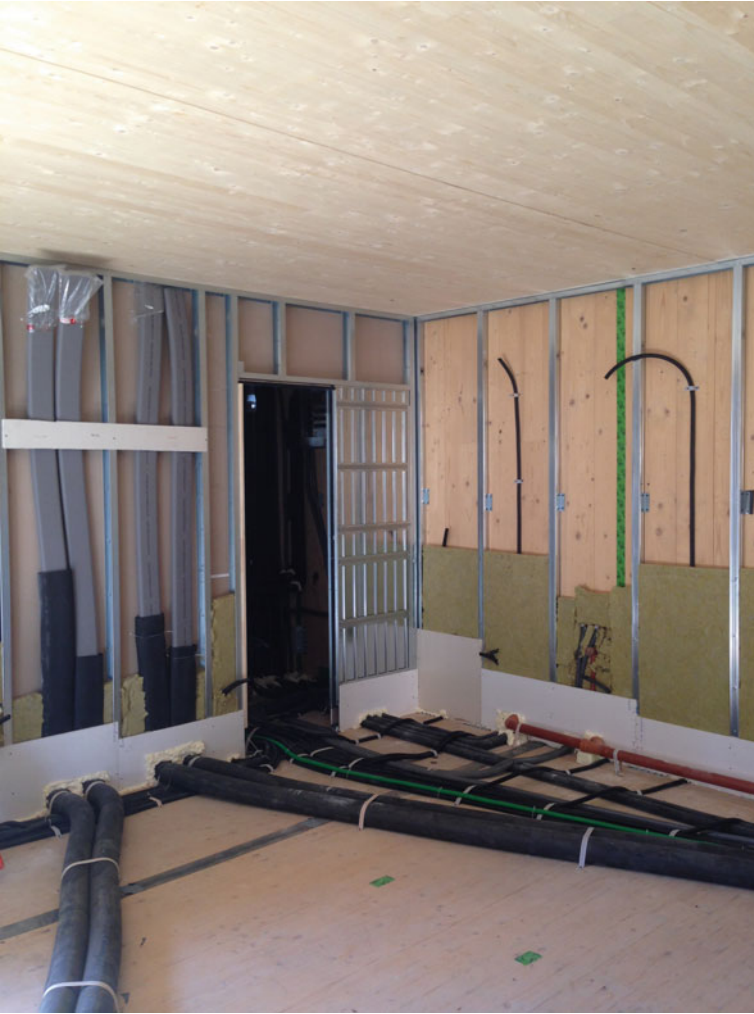
Fig. 9.15 Distribution of the technical systems in an apartment. The ventilation tubes that have a circular section on the interfloor slab and a smaller cross section when they are introduced into the internal wall
