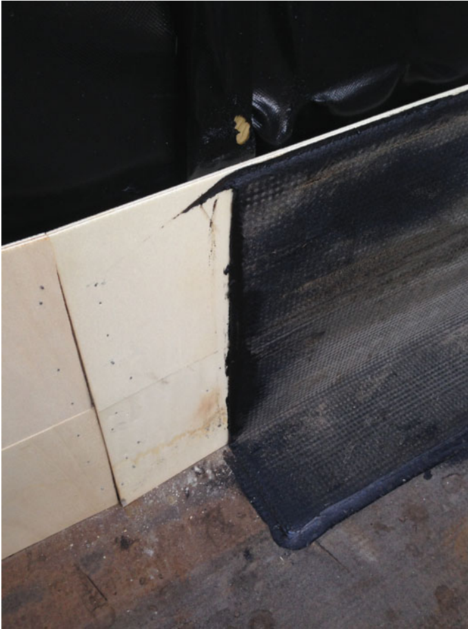
Fig. 5.7 Waterproofing in the point of contact of the wall with the terrace. The waterproofing sheath will be covered by an aluminium slat
