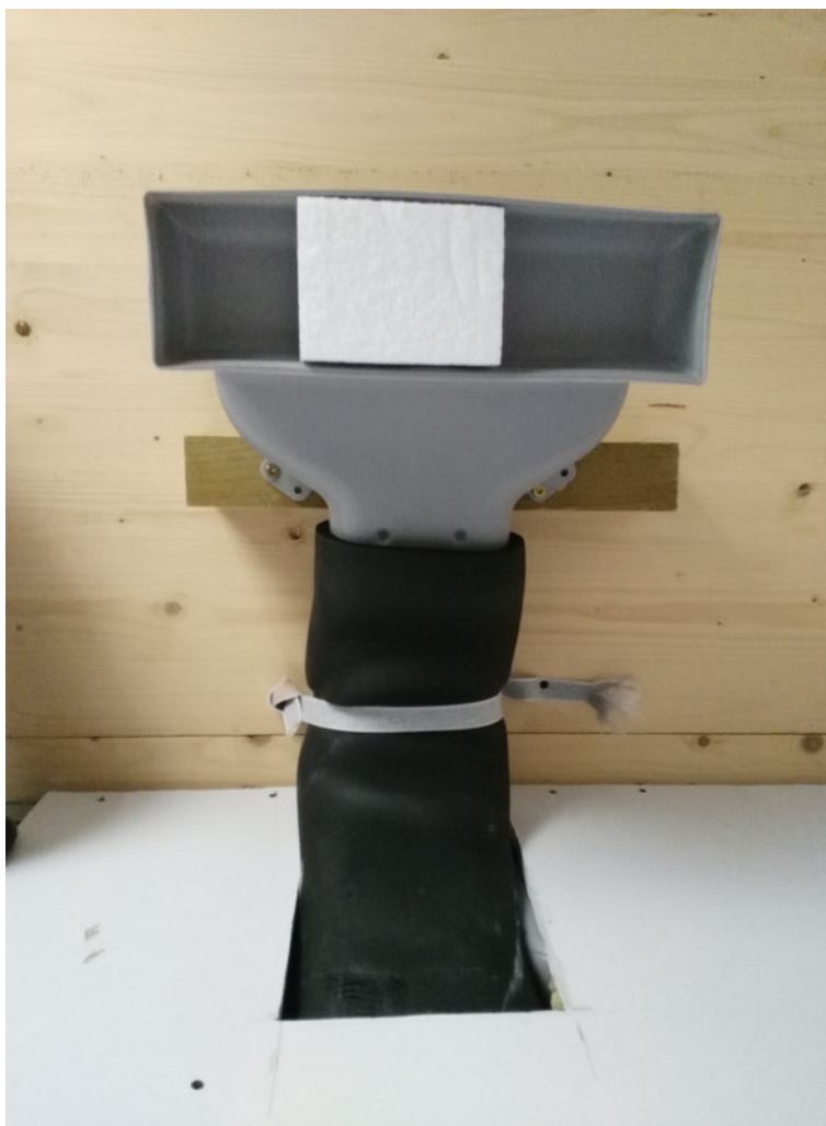
Fig. 9.10 Detail of a delivery air vent placed in a living room
