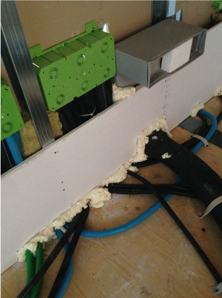
Fig. 9.13 Electrical boxes and delivery vent of the mechanical ventilation arranged in an internal wall. The polyurethane foam has the sole function of fastening
