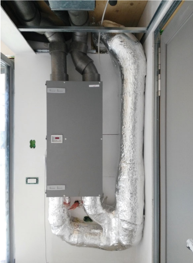
Fig. 9.3 Ventilation unit positioned vertically. The two tubes that connect the unit to the external environment were individually insulated with 8.5 cm thick insulation
