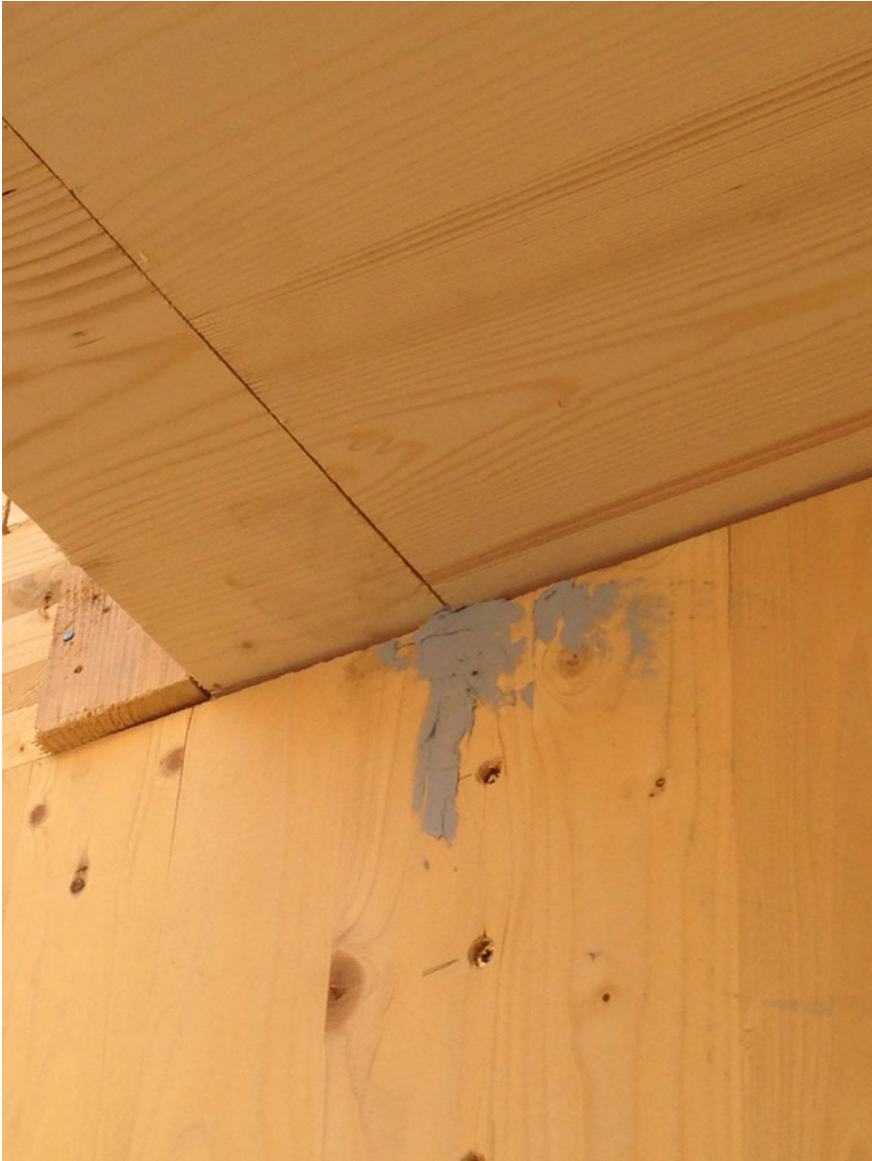
Fig. 8.8 Silicone injection in the presence of the joints of the horizontal panels of the floor slabs, carried out before the application of the sealing tape
