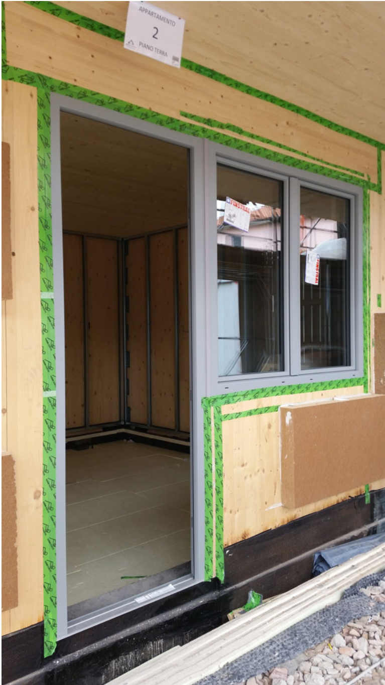
Fig. 8.9 Taping of the system of door and window frames with coupled window and entrance door
