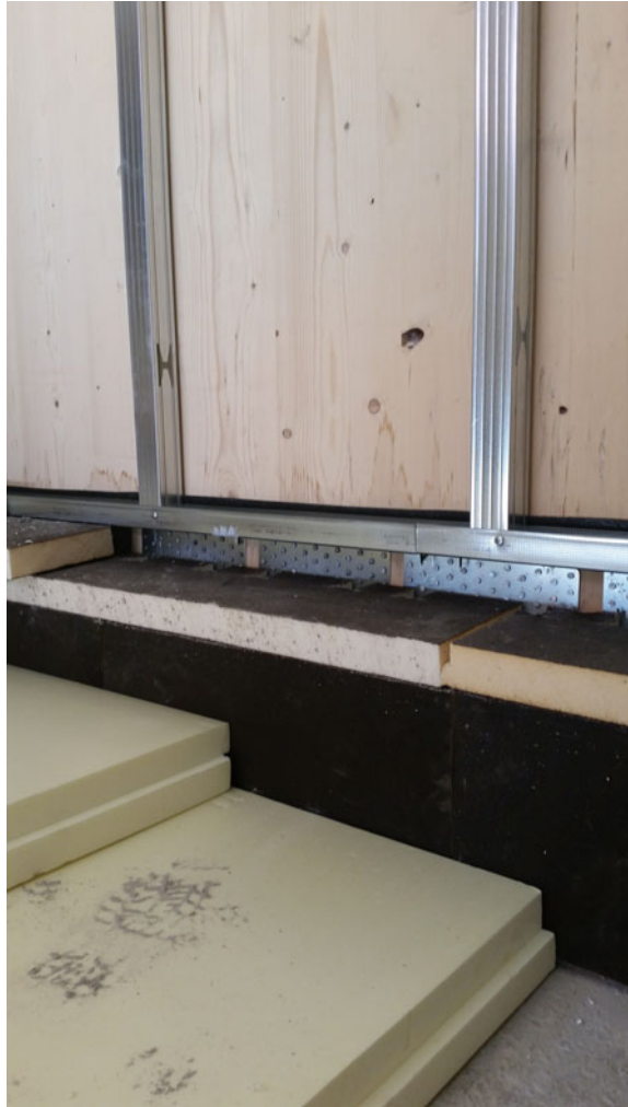
Fig. 7.12 Protection of the node with polyurethane panels having an impermeable surface (black)
