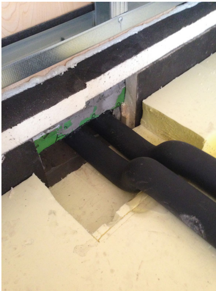
Fig. 9.12 Interferences between the two hot water pipes and the insulation of the ground slab. The interference will be resolved by placing insulation that has been specially shaped to adhere to the section of the tubes, all of it to be sealed with injections of polyurethane foam
