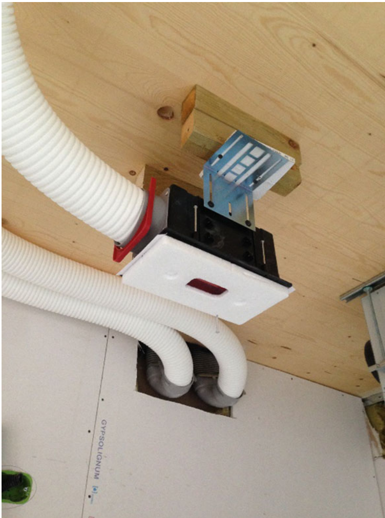
Fig. 9.5 Detail of a recovery vent located in a bathroom
