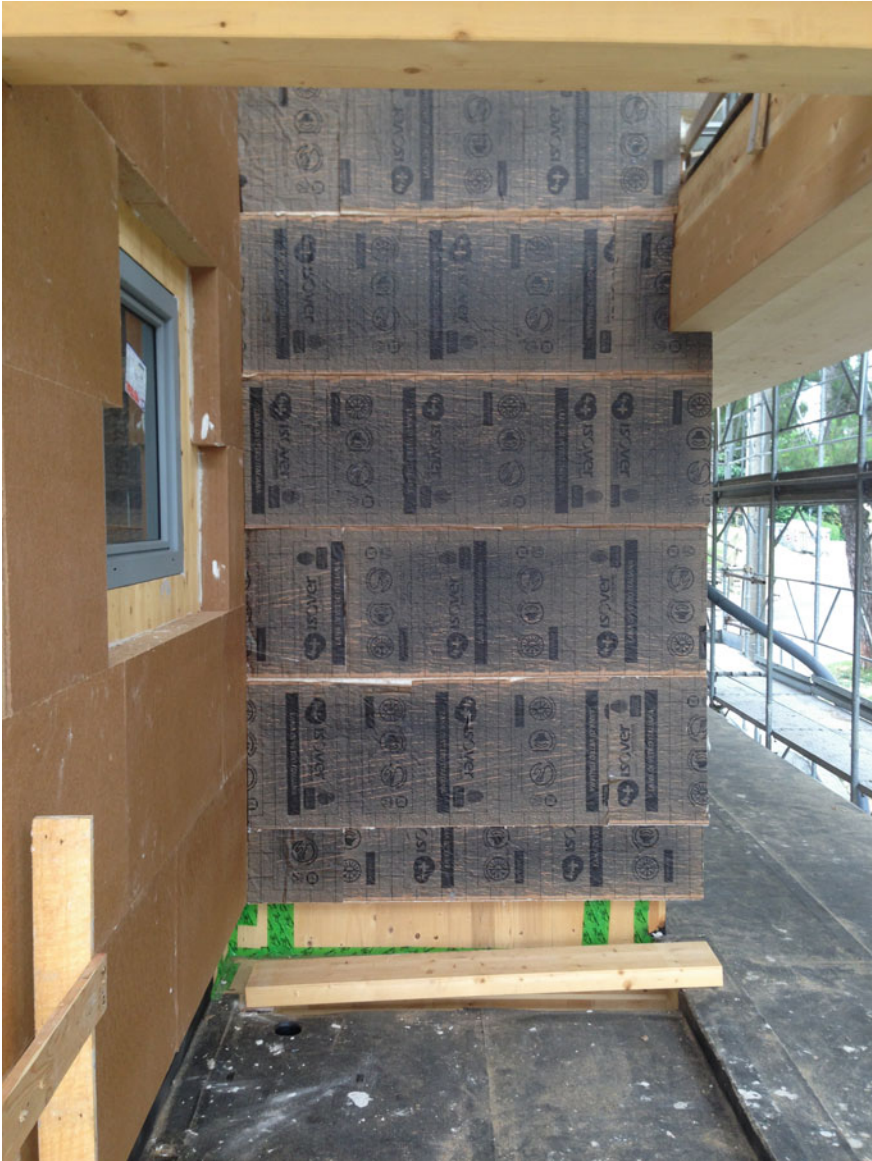
Fig. 5.4 Fibreglass with water vapour barrier towards the outside (incorrect installation)
