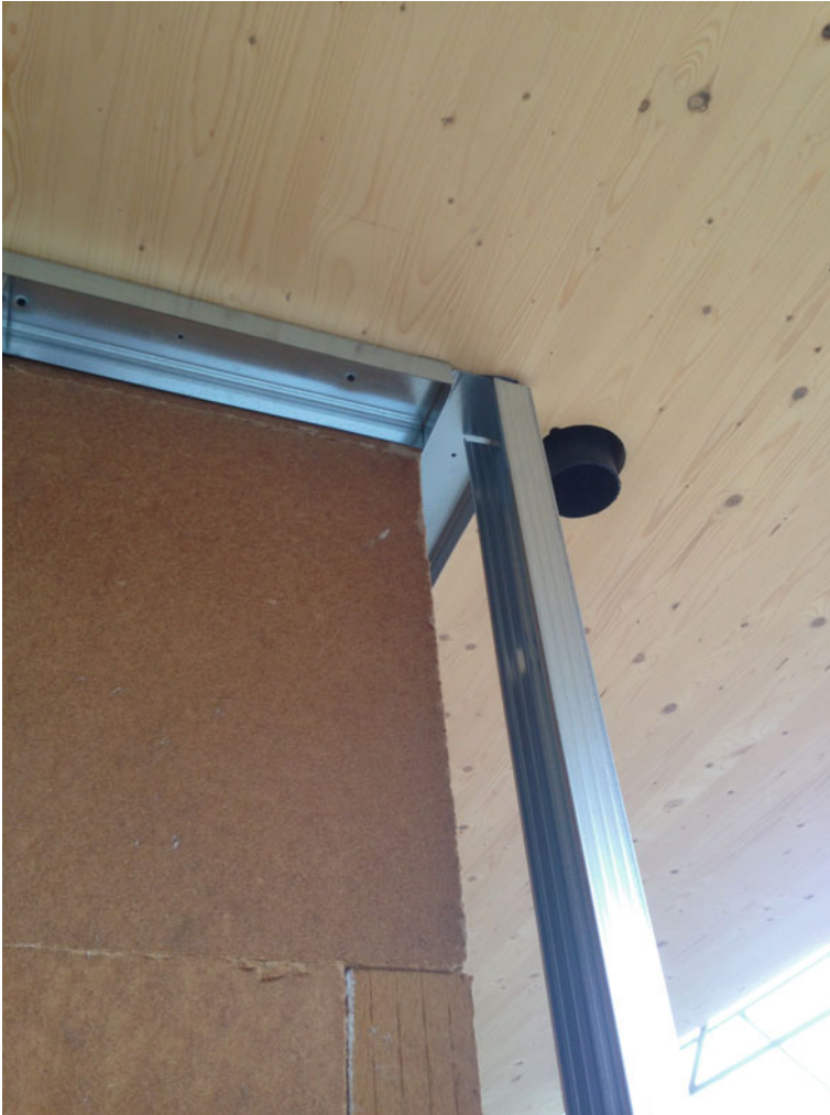
Fig. 5.15 Application of the studs on the panel in CLT of the terrace
