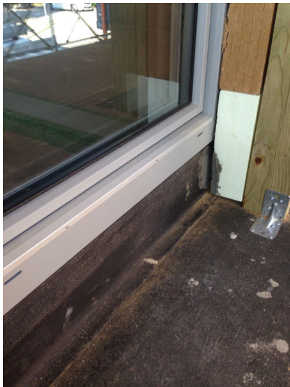
Fig. 7.37 Lower installation of the French windows onto an element in larch wood, protected by a waterproof membrane
