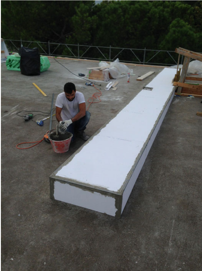
Fig. 7.1 Protection of the thermal bridge caused by a metal beam placed in the roof: the beam was insulated and coated with panels in fibre cement
