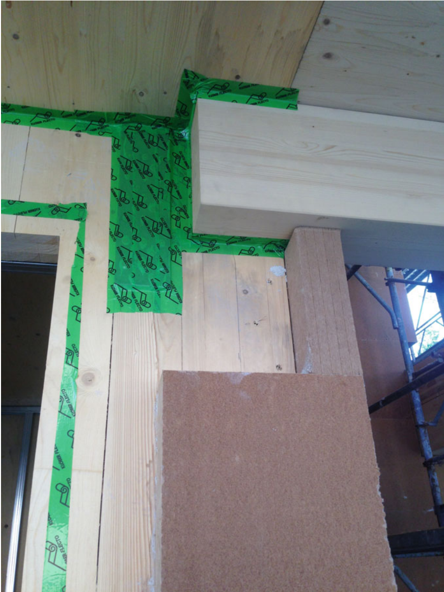
Fig. 8.6 Taping in the presence of the anchoring plate with holes that pass through and protruding wooden beam
