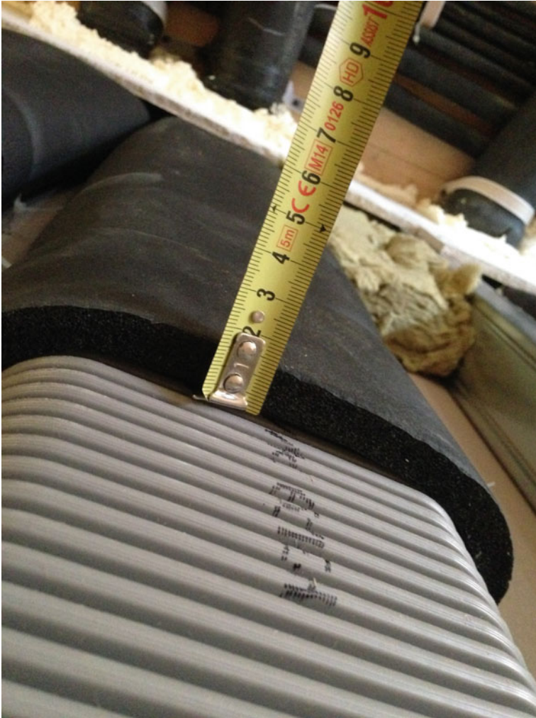
Fig. 9.9 Insulation of a flat air delivery tube placed within a false wall
