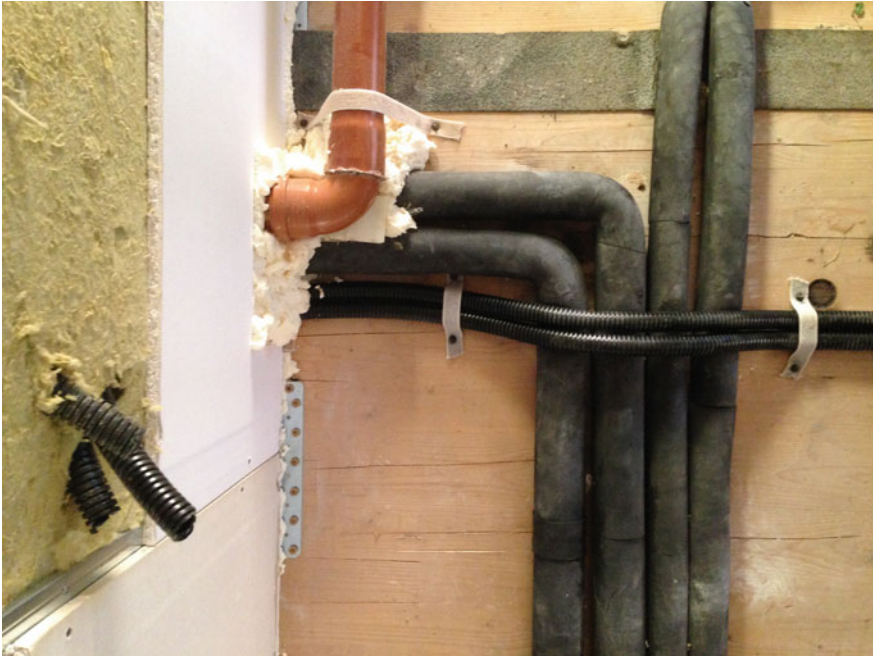
Fig. 9.11 Hot water pipes insulated with a thickness equal to twice the diameter of the pipe. The pipes are surmounted by a cable duct (black) and by a wastewater drainage pipe (orange)
