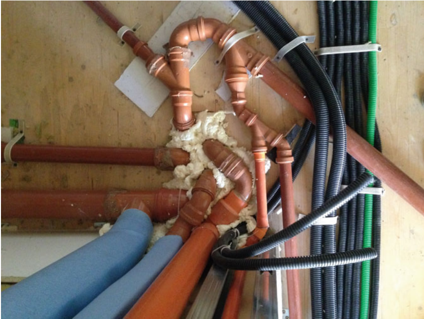
Fig. 8.16 Polyurethane foams applied in the hole of the traversing of the panel in CLT of the interfloor slab to ensure good airtightness between the different apartments. The requirement will be further enhanced by the subsequent laying of the lightened screed and the cement screed that will integrally cover the plants
