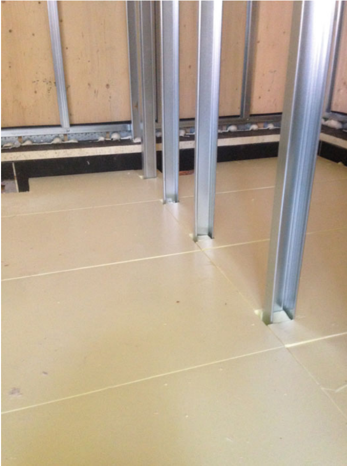
Fig. 5.29 Ground slab after the installation of the insulating panels. All the interstices between the panels will be subsequently filled with polyurethane foam
