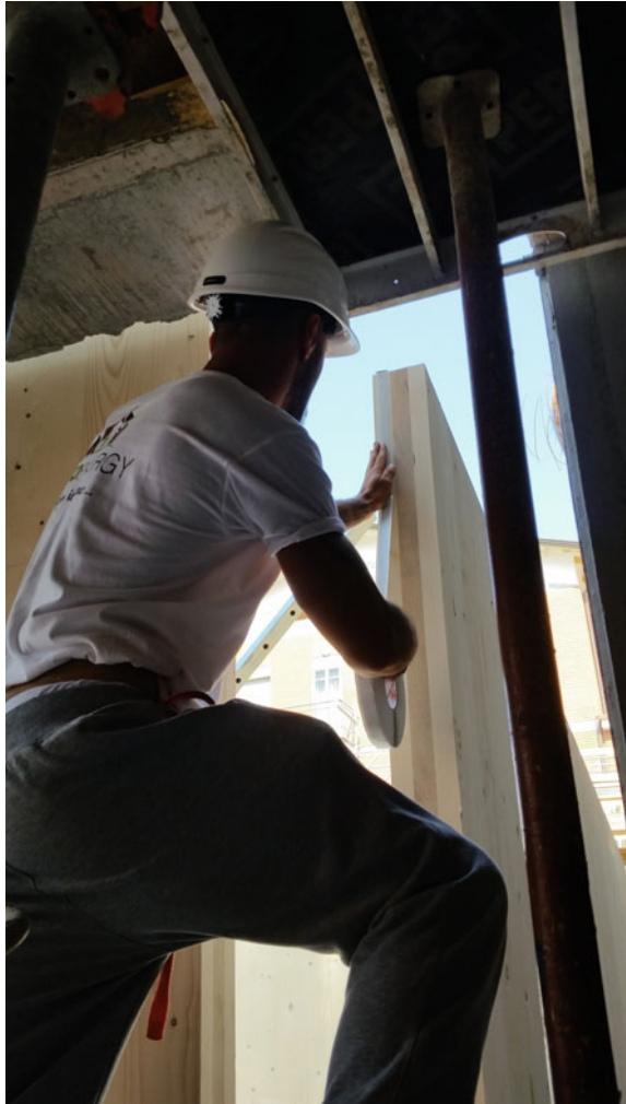
Fig. 4.26 Application of the butyl tape along the vertical joints of the panels in CLT
