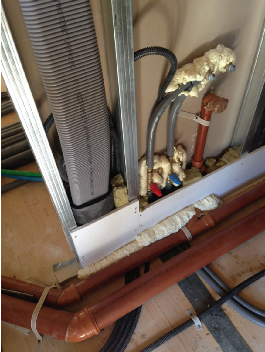
Fig. 8.13 Injection of polyurethane foams in the holes of the traversing of water tubes (internal side)
