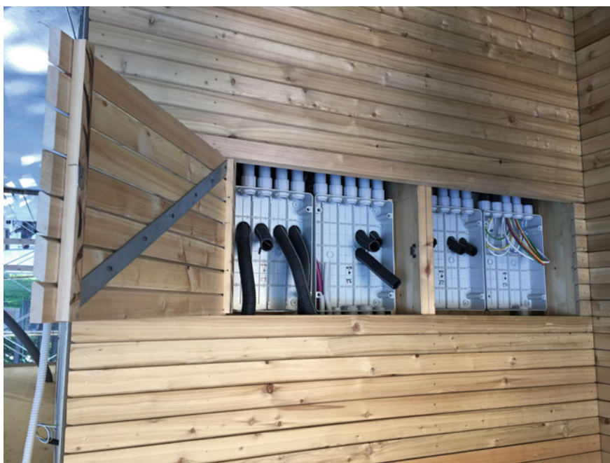
Fig. 9.21 Main distribution of the wiring situated outside of the heated envelope
