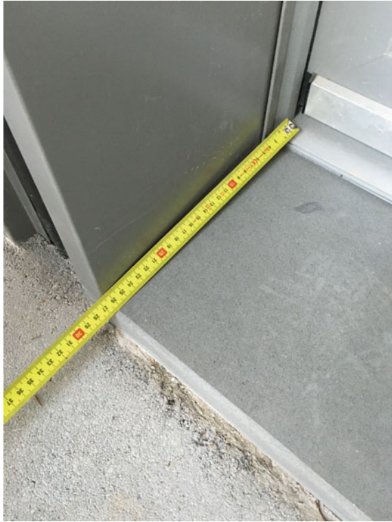
Fig. 7.41 Lower installation of the French door after the installation of the stone threshold
