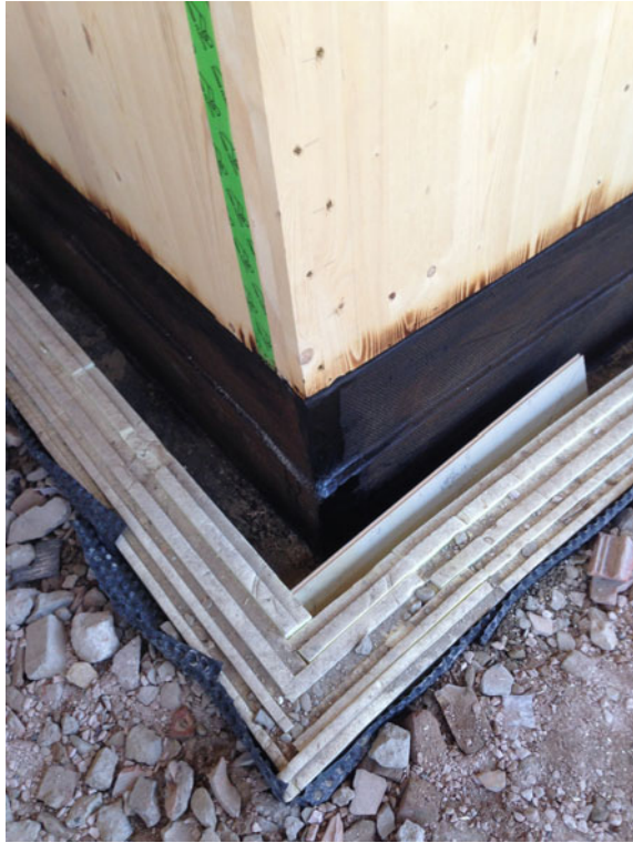
Fig. 4.35 Application of waterproofing sheath at the joint between the foundation kerb and the vertical panels in CLT
