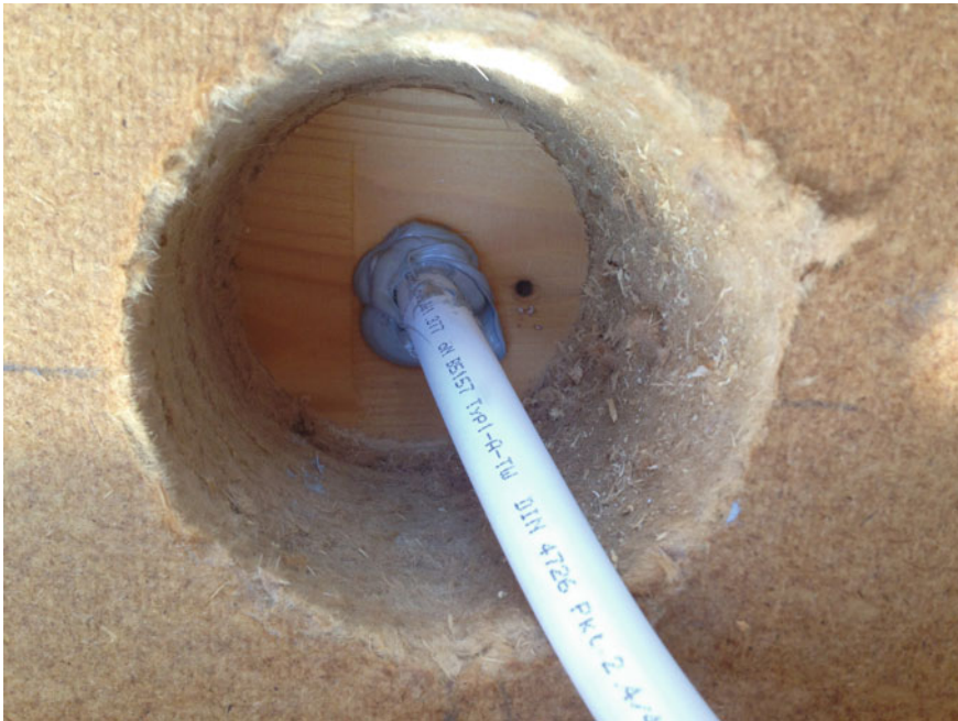
Fig. 8.12 Injection of silicone glues in the hole of the traversing of a water tube (external side)
