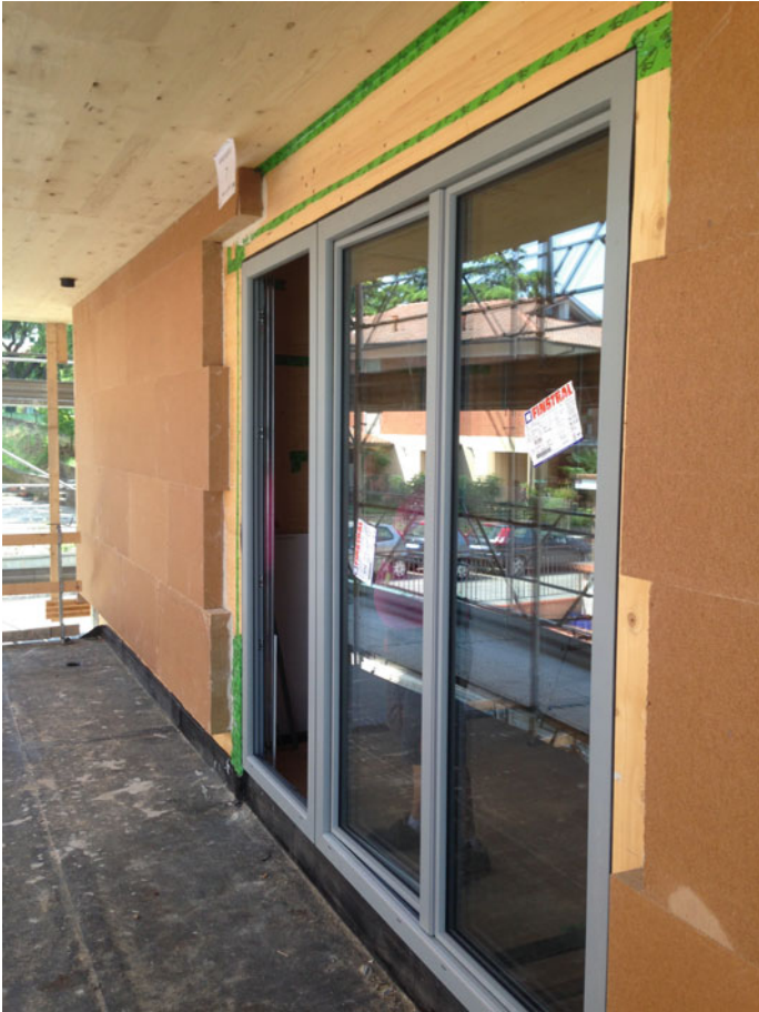
Fig. 5.33 French door integrated to the entrance door
