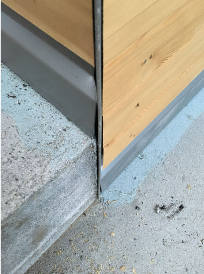
Fig. 5.26 Difference in height between the terrace floor slab and the terrace. The surfaces will be subsequently treated with resin flooring
