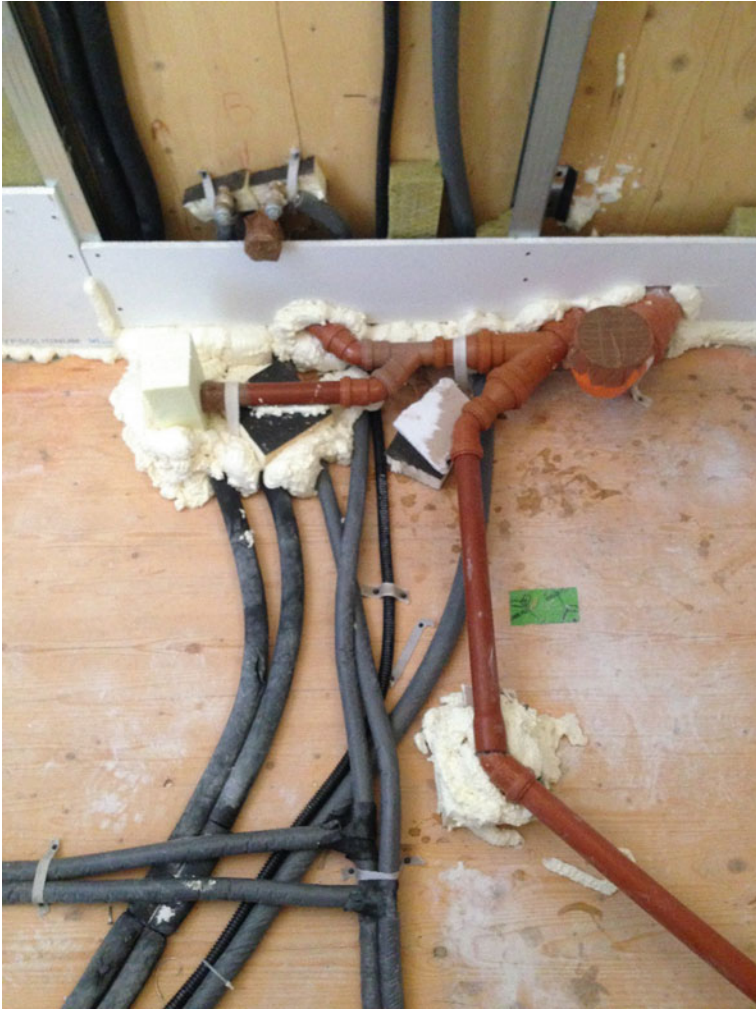
Fig. 9.2 Passage of the wastewater drains through the panel in CLT of the interfloor slab
