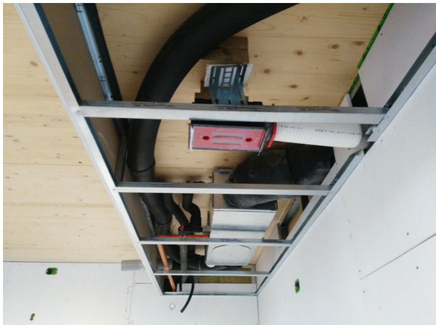
Fig. 9.8 Studio apartments are equipped with a shared ventilation system, while the ventilation unit with heat exchanger is located in the garage; each apartment has its own pre-heating controller, together with a recovery vent, placed within a false ceiling in plasterboard
