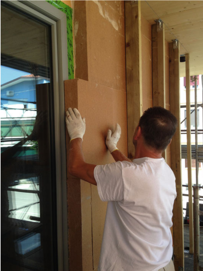
Fig. 5.31 Thermal insulation covers the frame of the fixture to limit heat loss
