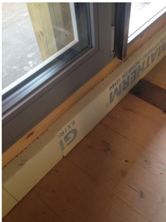
Fig. 7.38 Lower installation of the French door seen from the internal side, where a 12-cm-high panel in XPS, with the same thickness of the screed, has been inserted
