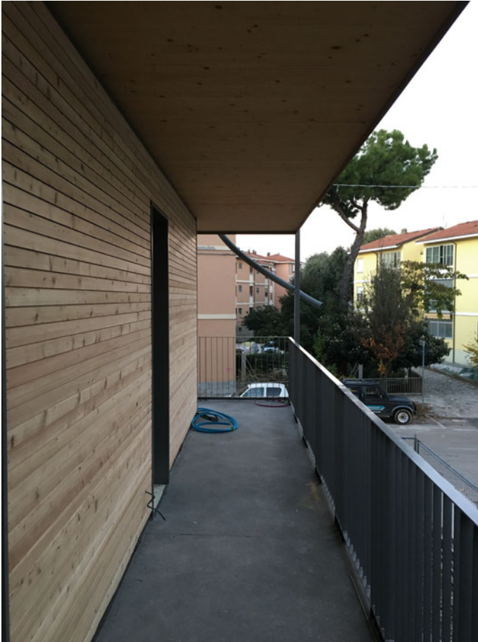
Fig. 7.17 Cement screed laid on the insulation in XPS, ready to receive the application of the resin flooring. The intrados of the upper terrace remains devoid of insulating, leaving the panel in CLT in view
