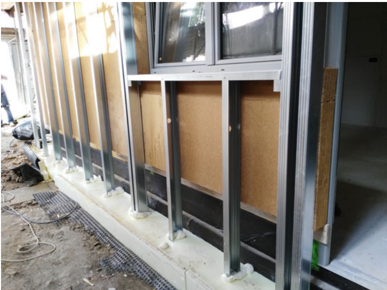
Fig. 7.6 Protection of the thermal bridge on the external side using panels in XPS. The interferences with the sheet metal structure are protected with injections of polyurethane foam
