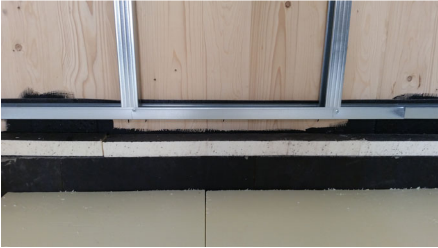
Fig. 7.7 Protection of the thermal bridge on the internal side using panels in polyurethane with impermeable surface (black)
