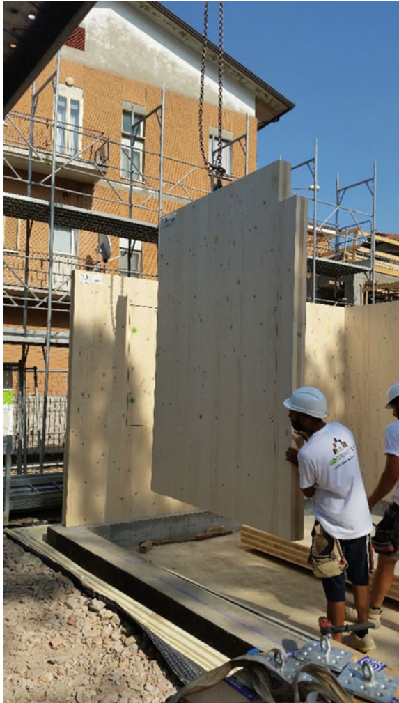
Fig. 4.12 Lifting of the panels in CLT and laying on the foundation's kerb
