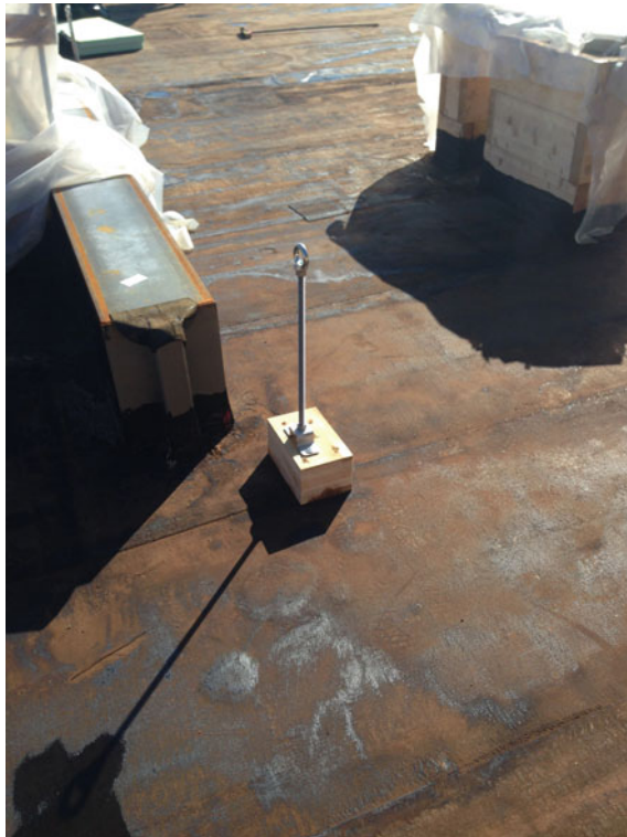
Fig. 7.44 Steel pin for the fixing of the line life anchored to the CLT
