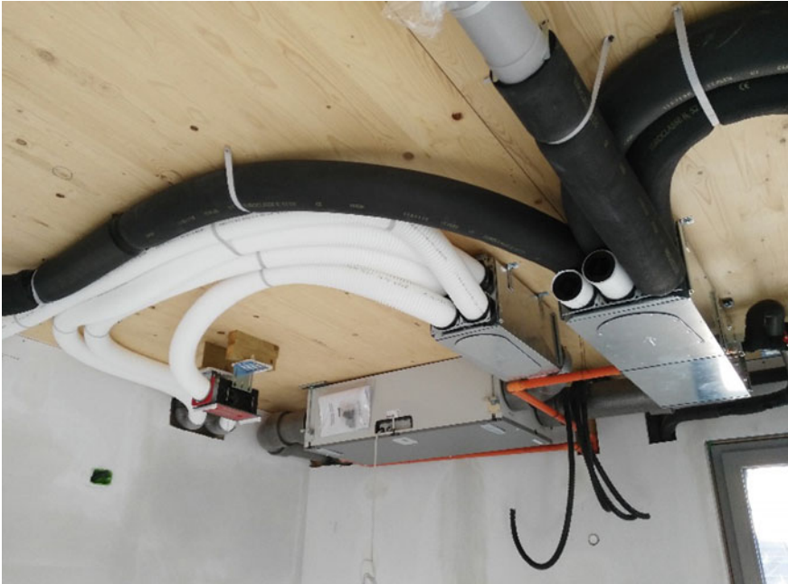
Fig. 9.6 Installation of the controlled mechanical ventilation system in the false ceiling of a kitchen consisting of: ventilation unit with heat exchanger, pre-heating controller and an air recovery vent. The insulation is placed in the delivery tubes (black) and in the tubes of the extracted and consumed air (grey)
