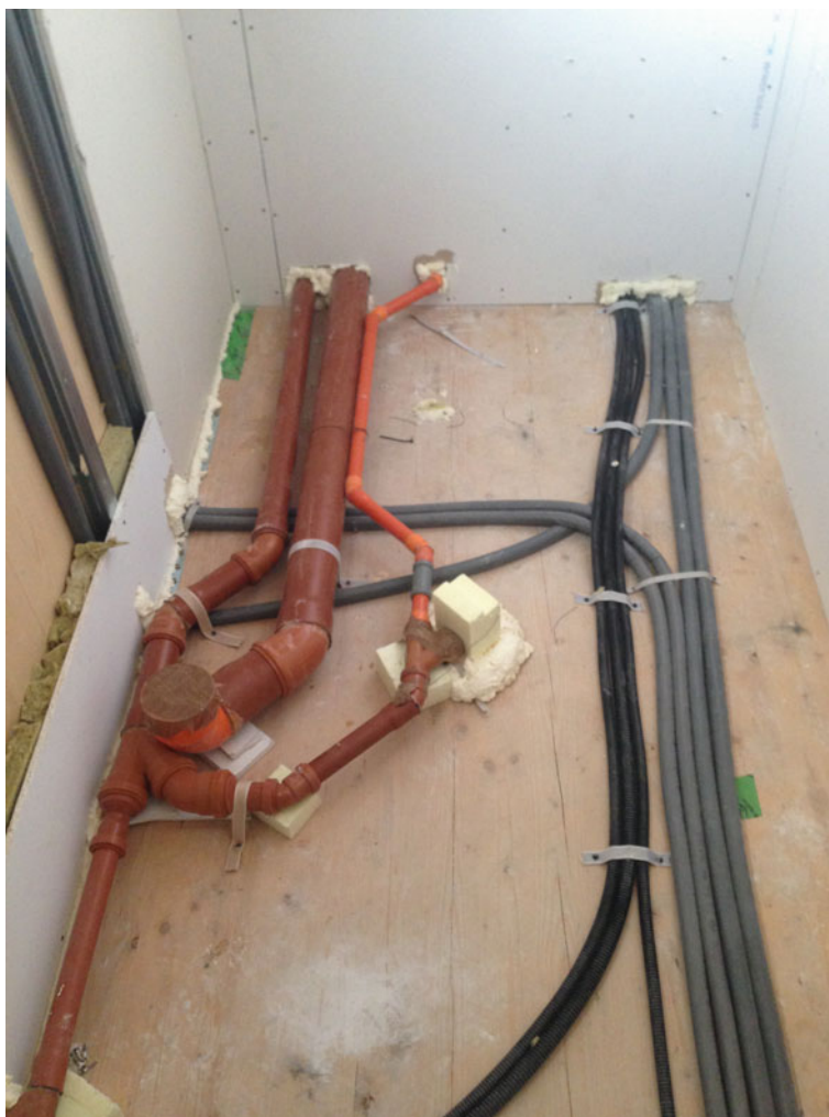
Fig. 9.14 Interfloor slab with wastewater drainage systems (orange), cable ducts (black), cold water pipes (grey)
