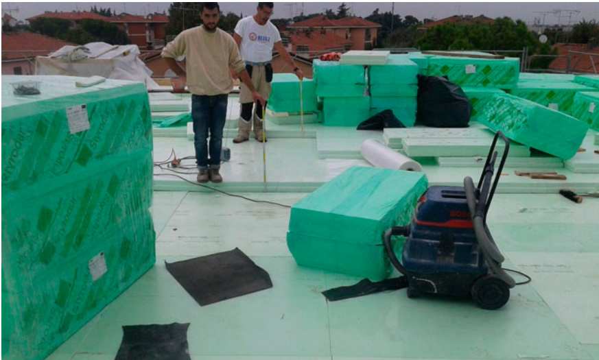
Fig. 7.21 Insulating panels in XPS laid in a uniform manner over the entire surface area of the roof for a total thickness of 32 cm
