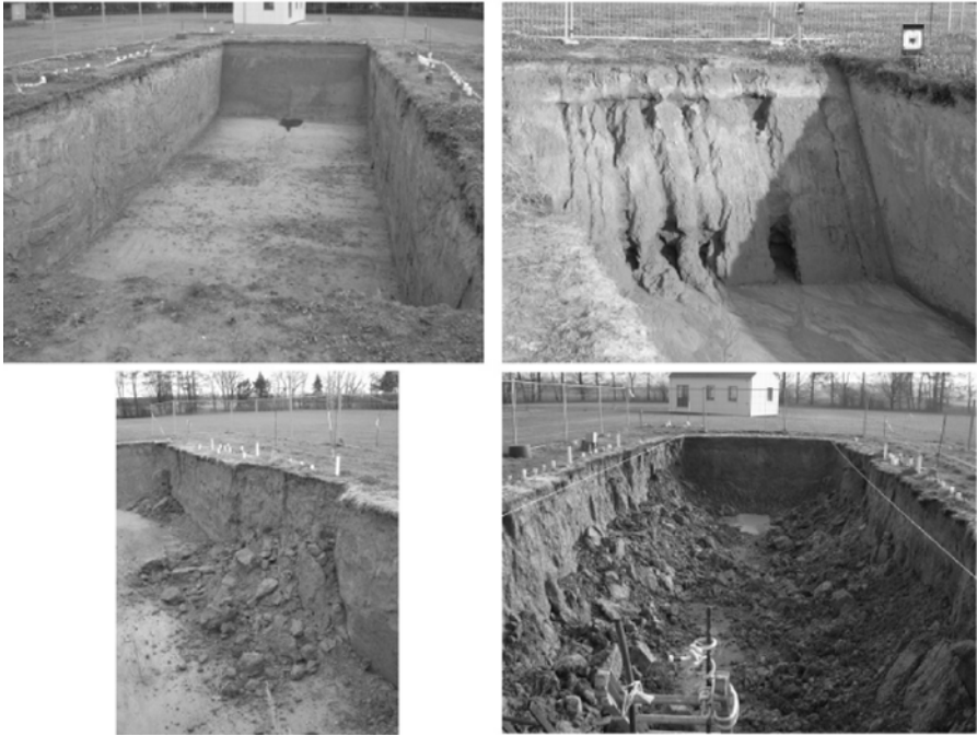
Fig. 8. Upper left: June 2004 – after excavation of the test trench; Upper right: first localised failures (January 2005); Lower left: eroded inclined sides; Lower right: generalized failures (February 2005)
