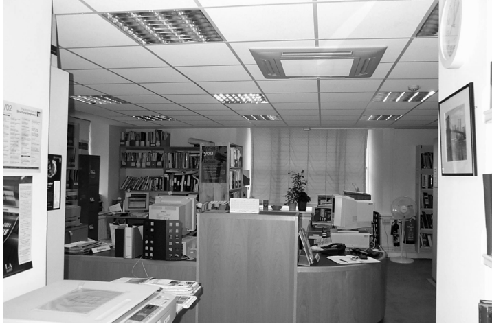
Figure 2.77 Illustration of a typical retrofit lighting scheme where little attention has been paid to the varying requirements of the space
