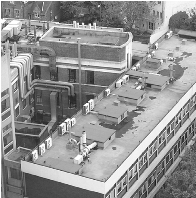
Figure 2.75 Retrofit of condenser units on a roof can increase roof clutter
