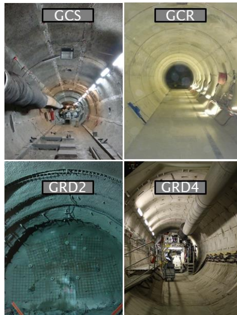
FIGURE 2. The four excavated drifts dedicated to structure influence study (parallel to the major in situ stress direction)
