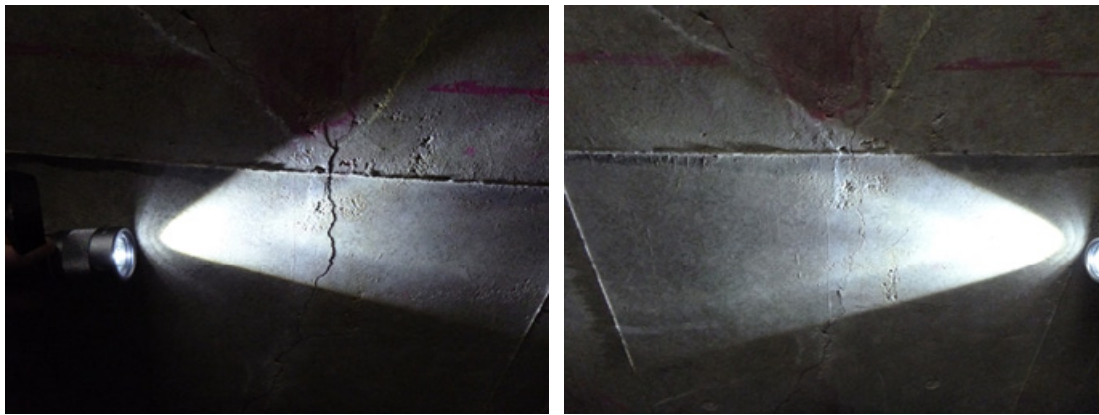
(a) Light from the span center (b) Light from the hunch side → Same crack is shoot, but shade appears only in (a) because of the gap.
