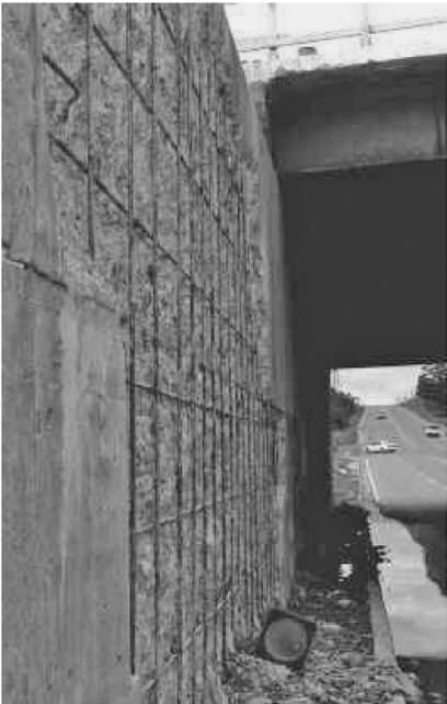
FIGURE 3.7 Photo of corroded abutment bridge wall.
