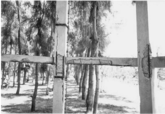
FIGURE 3.9 Photo of cracks on columns and beams.
