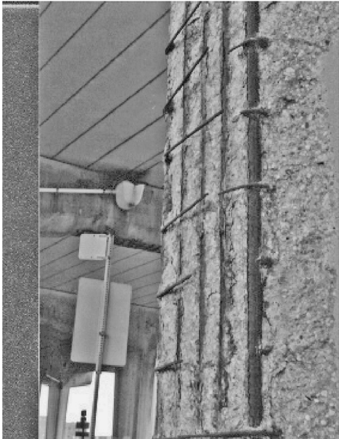
FIGURE 3.6 Photo of corrosion in concrete.
