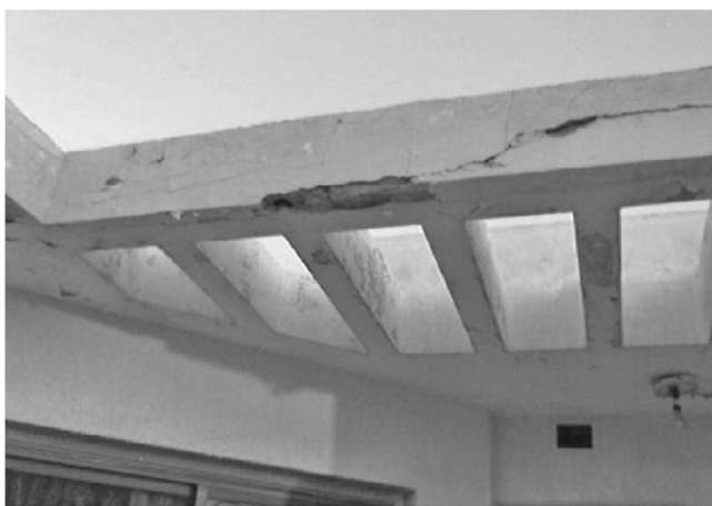
FIGURE 2.1 Deterioration in a reinforced concrete beam.
