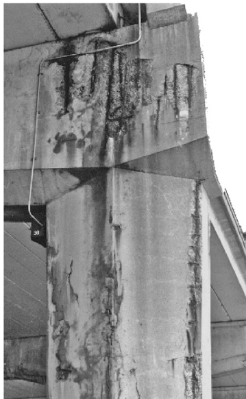
FIGURE 4.3 Brown spots on bridge column and girder.
