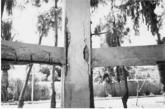
FIGURE 3.8 Photo of cracks in columns of elevated water tanks.
