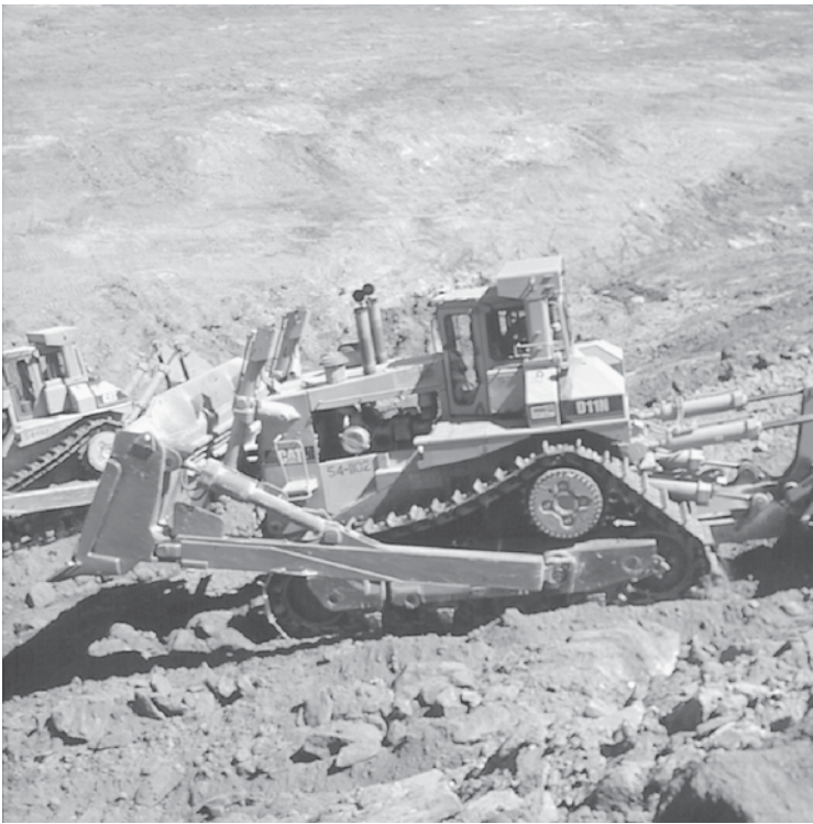
FIGURE 18.6. D-11 CAT Working on a Major Highway Job. Is an Inspector or a Construction Engineer Qualified to Inspect such Equipment?
