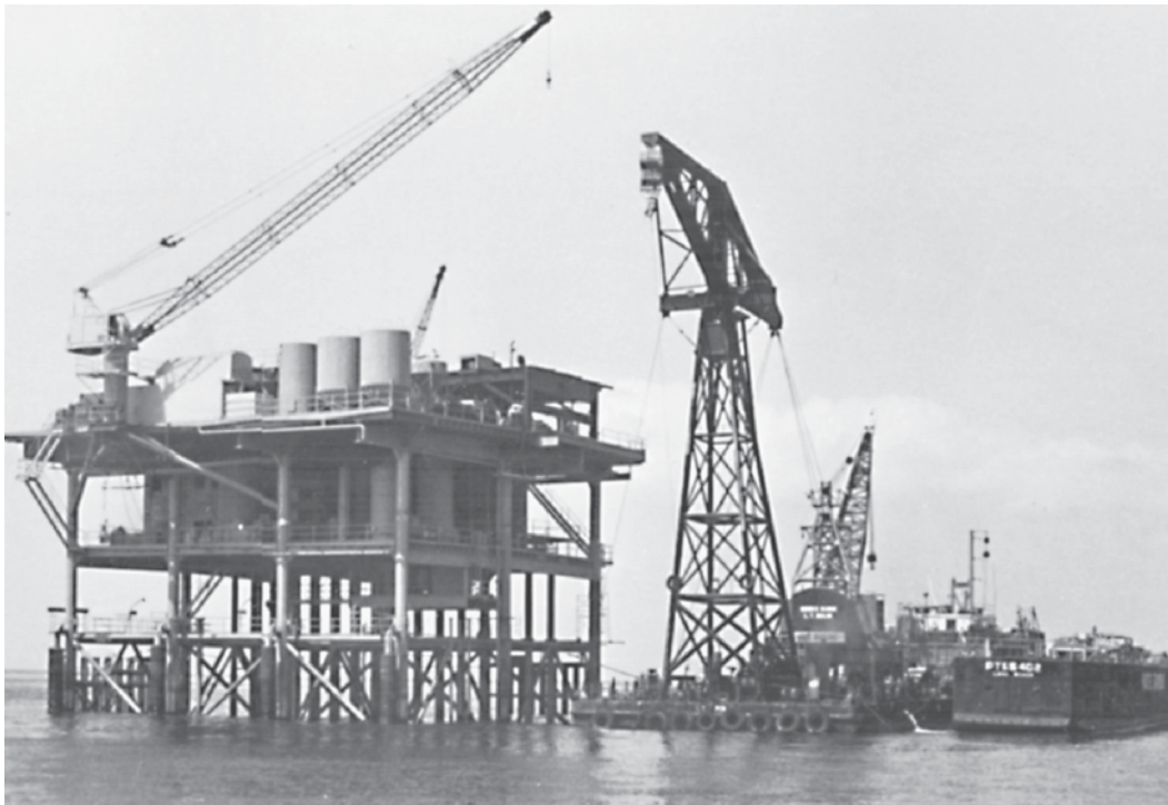
FIGURE 18.1. Offshore Construction Presents Special Problems for Access to the Work by the Inspectors, as well as Increased Insurance Risks.
