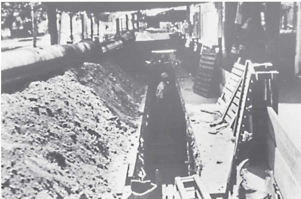
FIGURE 9.3. Photographic Documentation of an Imminent Hazard.
