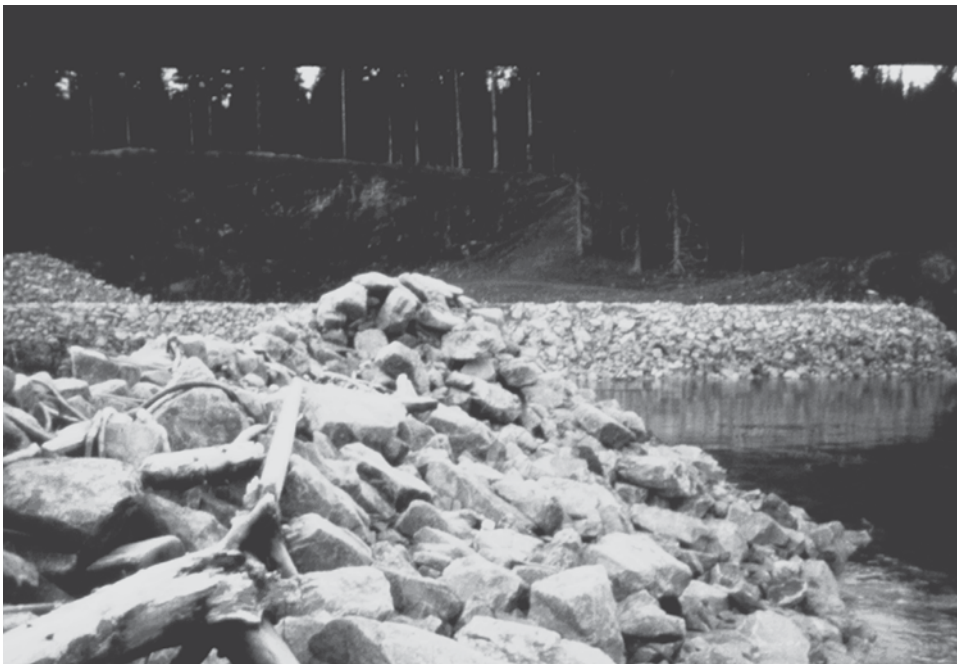
FIGURE 21.1. Failure of Improperly Designed Breakwater That Was Built in Accordance with Plans and Specifications.
