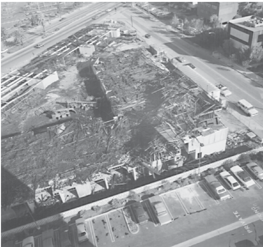
FIGURE 20.2. Fire Damage to a Project under Construction. Owner Suffered Total Loss Due to Failure to Include Policy Provisions in the Construction Contract.
