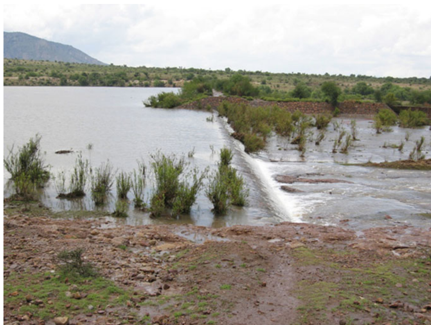
Fig. 9.20 Los Izquierdo Dam in 2010, during flooding caused by Hurricane Alex (Conagua SISP 2016)
