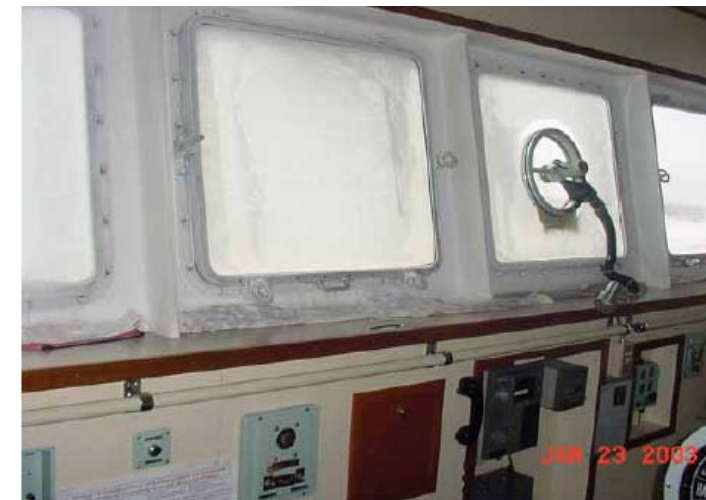
Figures 9.1B – Deficient wheelhouse heating combined with a high rate of humidity
