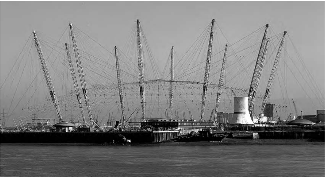
3.23 The Millennium Dome. Cable net before the textile covering was put on.
