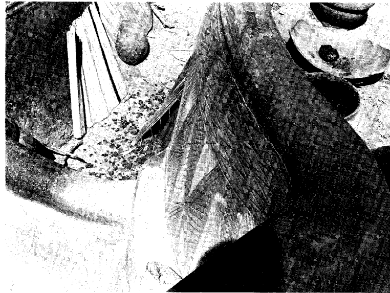
Fig. 24: A portion of a flat mud roof in a Nankansi compound near Sirigu showing two built-in pots without bottom acting as ventilation and light opening, 1972.
