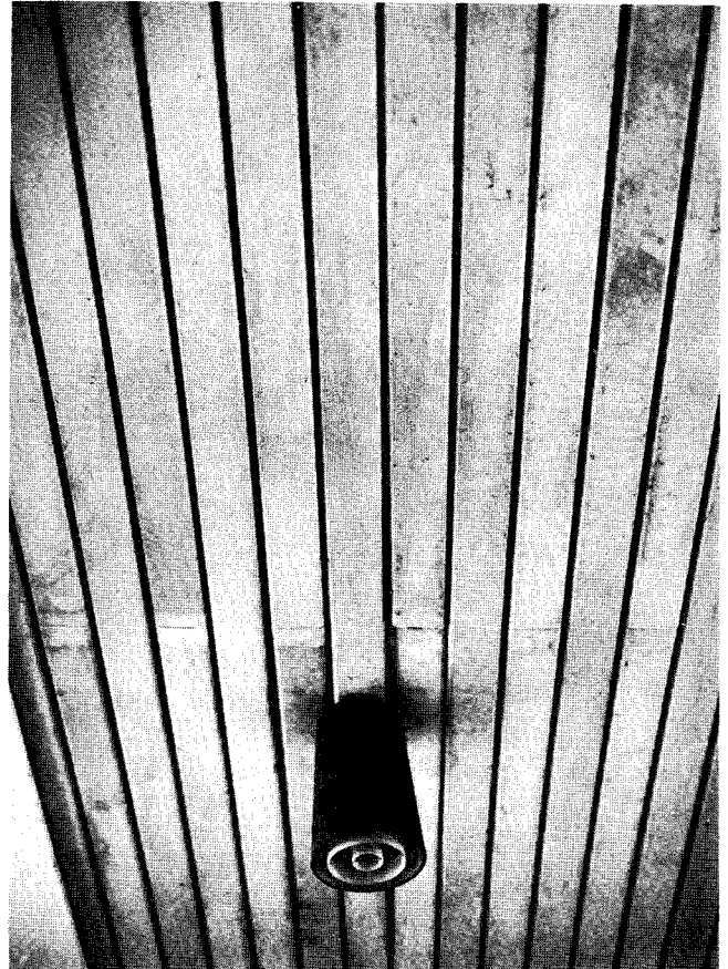
For Fig. 351: Aluminium strip ceiling of the Conference Room, Great Hall, U.S.T., 1982. Architects: GERLACH & GILLIES REYBURN.
