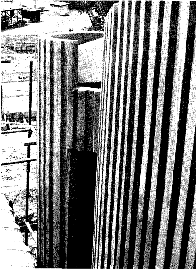
Fig. 296: Patterned concrete finish on the walls of the Members' Lobbies, Parliament House extensions, Accra, 1970.
