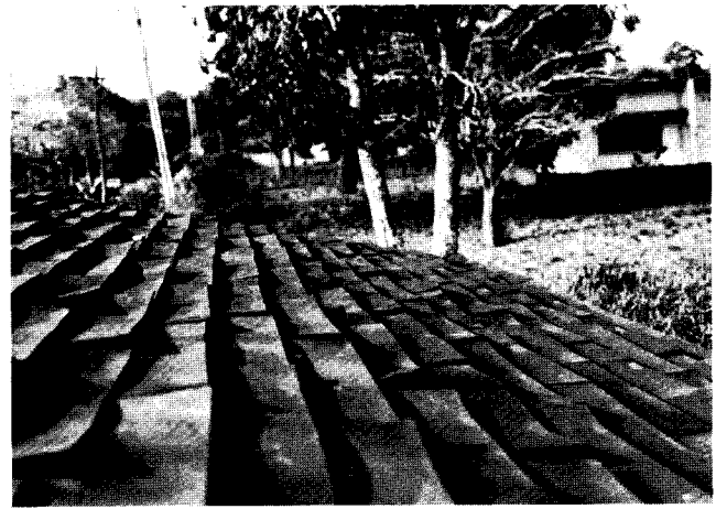
Fig. 201: Experimental bagasse – reinforced phenolic composite roofing shingles on a kiosk at the Council for Scientific and Industrial Research headoffice in Accra, 1981.
