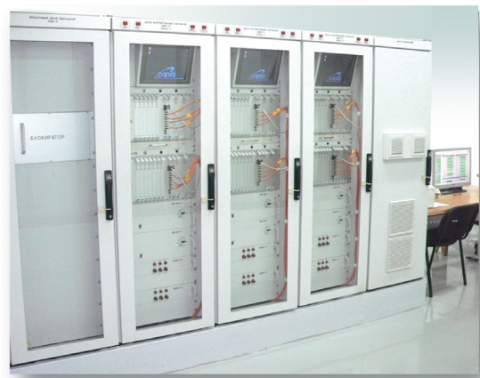
Figure 9. Software-hardware complex of reactor power control, unloading, limitation and accelerated preventive protection system
