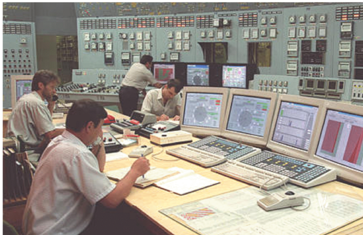
Figure 3. General view of the SPDS at the main control room
