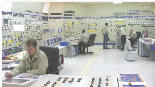
Figure 4. Main control room at Rovno NPP
