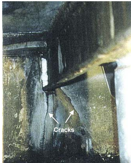
Fig. 8. Cracks at end cross girder web
