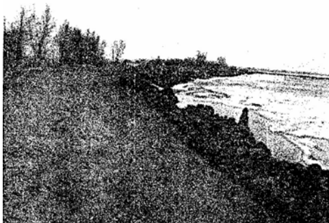
Fig.1 the picture for frost damage of dyke
