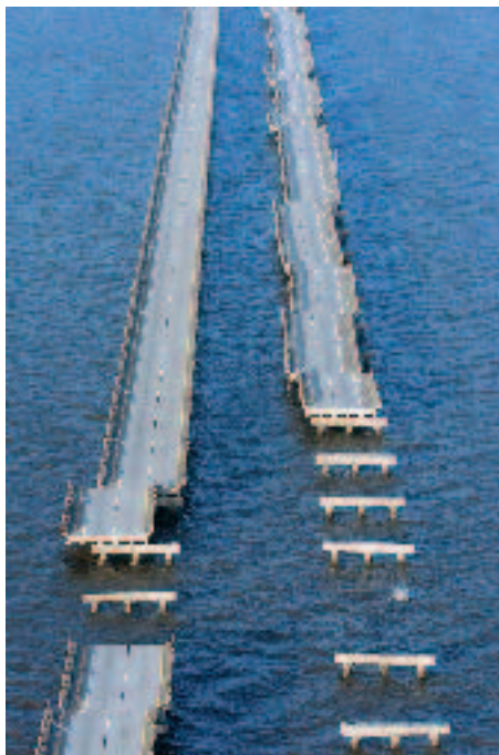
Figure 1.9 Failure of the Escambia Bay bridge in Pensacola, Florida, during Hurricane Ivan in September 2004.
