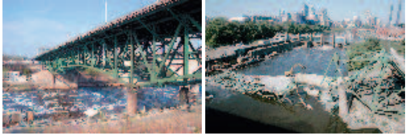
Figure 6.23. Failure of the Interstate 35W bridge in Minneapolis, Minnesota. This bridge opened to traffic in 1967 and collapsed without warning during the evening rush hour on August 1, 2007, killing 13 people and injuring over 100 more. The National Transportation Safety Board's (NTSB's) investigation determined that some of the gusset plates were undersized and that failure of some of these initiated collapse of the bridge. One of the criticisms of this bridge's design is that it was statically determinate, and hence failure of one member or connection is sufficient to cause collapse of the entire structure.
