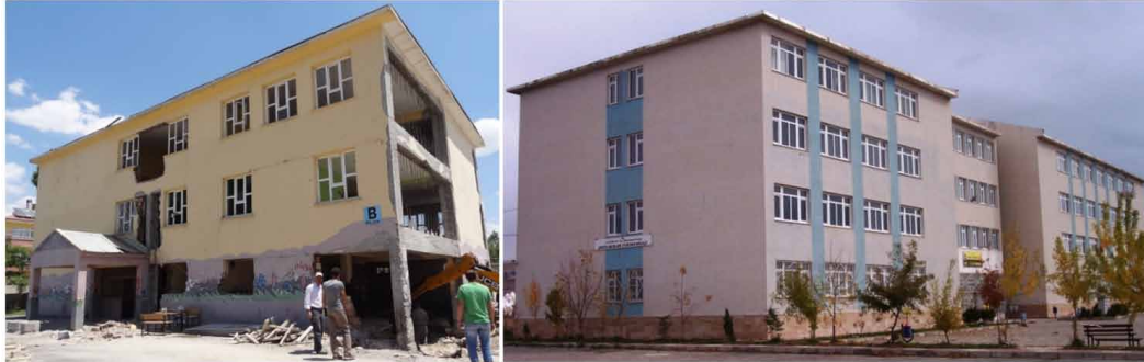
Figure 1. Typical small- (left) and large-scale (right) RC school buildings in Turkey Pictures taken by B.Taskin
