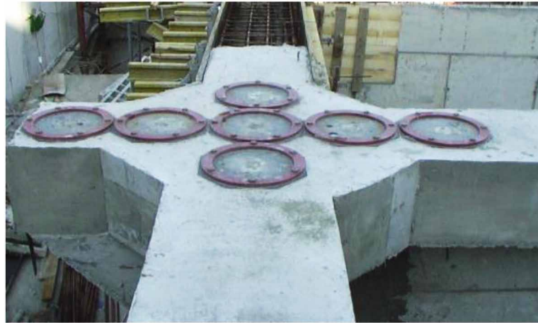
Figure 5. The concrete under the sockets of small size isolators is casted without difficulties and with high quality
