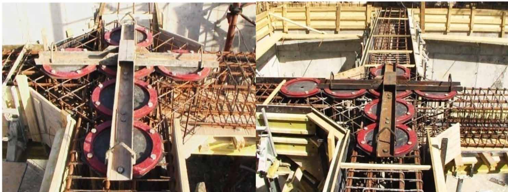
Figure 4. Precise fixing of the isolator's sockets in the design position using special conductors
