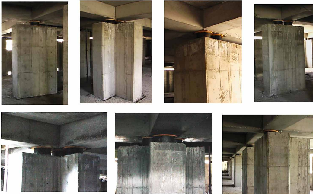
Figure 23. Types of the columns and examples on installation of rubber bearings' clusters in the basement of the 4-story base isolated hospital building “Vanadzor”
