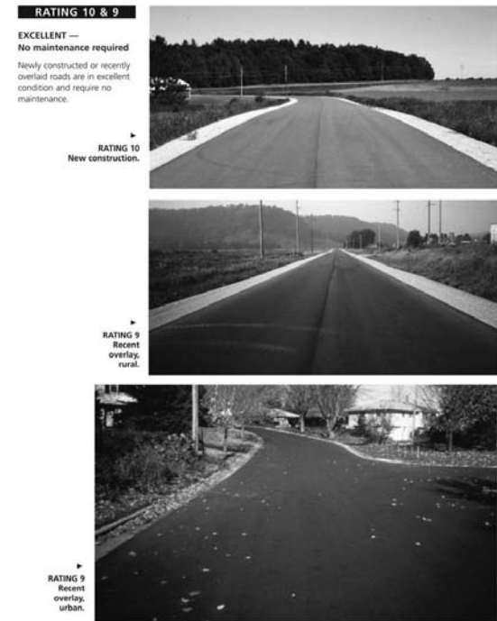
Figure 4-11. Method of Assigning a Composite Condition Index Using PASER (Wisconsin Transportation Information Center 2002)
