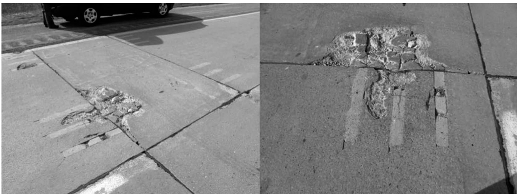
FIGURE 18.14 The I-675, Michigan PCP rehabilitation project with deteriorated panels before replacement. (Courtesy of National Academy of Sciences.)
