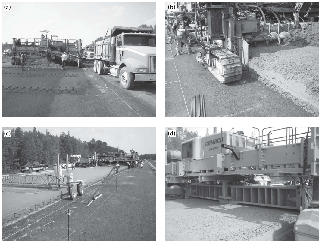
FIGURE 17.6 Typical paving train showing (a) slipform paver, (b) auger, (c) finishing and texturing unit, and (d) striker bar. (Courtesy of Wouter Gulden, ACPA-SE Chapter, Duluth, GA.)
