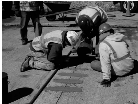
FIGURE 18.3 The DBR method which is used in a variation of the intermittent repair technique with dowel bars installed and grouted. (Courtesy of National Academy of Sciences.)
