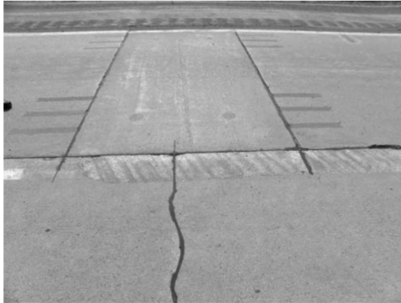
FIGURE 18.15 A well-performing panel at the I-675 project in Michigan. (Courtesy of National Academy of Sciences.)
