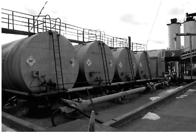
FIGURE 13.11 Asphalt storage tanks. (Courtesy of Matthew Teto, All States Asphalt, Sunderland, MA.)
