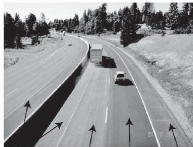
Recycled shoulder Recycled no.1 lane Mill and fill no.2 lane Recycled shoulder
