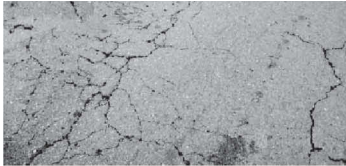
Cracks in existing pavement
