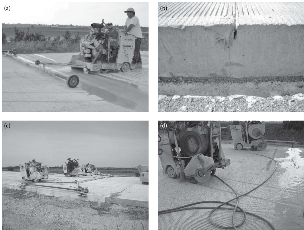
FIGURE 17.16 (a–d) Joint sawing operations in PCC pavements. (Courtesy of Wouter Gulden, ACPA-SE Chapter, Duluth, GA.)
