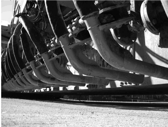
FIGURE 17.7 Typical slipform vibration system. (Courtesy of Robert Rasmussen, Transtec Group Inc., Austin, TX.)
