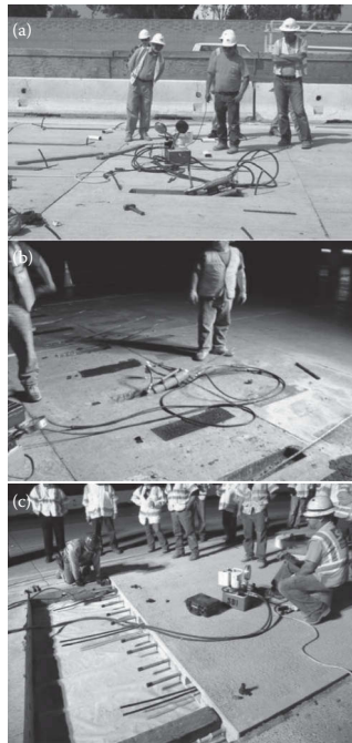
FIGURE 18.6 Installation of three versions of PPCP systems with stressing pockets are shown (a) in central panel, (b) at expansion panel, and (c) with posttensioning performed at joint face. (Courtesy of National Academy of Sciences.)
