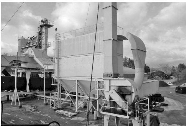
FIGURE 13.10 Baghouse. (Courtesy of Matthew Teto, All States Asphalt, Sunderland, MA.)
