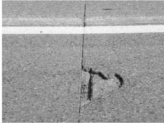
FIGURE 18.19 Spalling resulting from high steel location and steel corrosion observed at the intermediate transverse joints at some locations. (Courtesy of National Academy of Sciences.)
