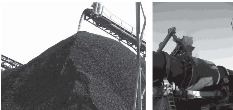
FIGURE 13.9 RAP stockpile and RAP feeding system in a drum plant. (Courtesy of Robert Frank.)
