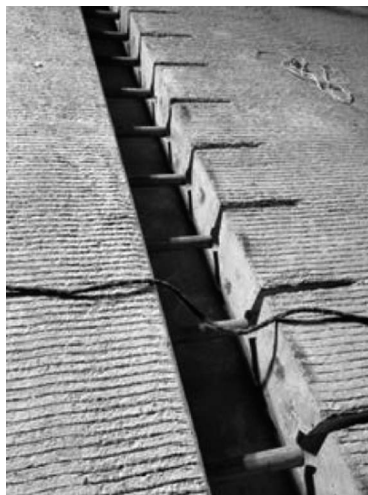
FIGURE 18.10 Embedded dowel bars being slid into the teardrop-shaped slots. (Photo Courtesy of Shiraz Tayabji, Applied Research Associates, Inc.)
