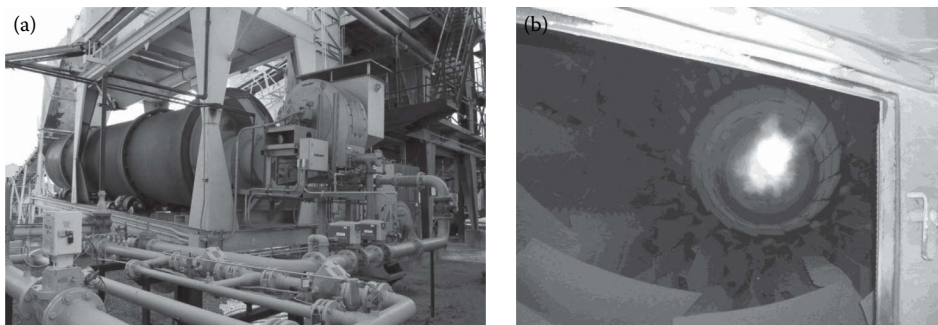
FIGURE 13.5 (a) Dryer drum with burner and (b) inside of drum. (Courtesy of Matthew Teto, All States Asphalt, Sunderland, MA.)
