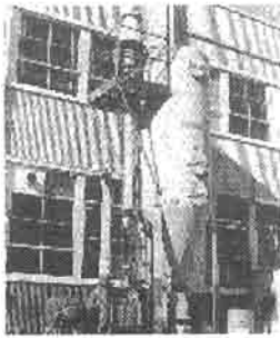
(c) Ground-level installation with a single baghouse air cleaner.
