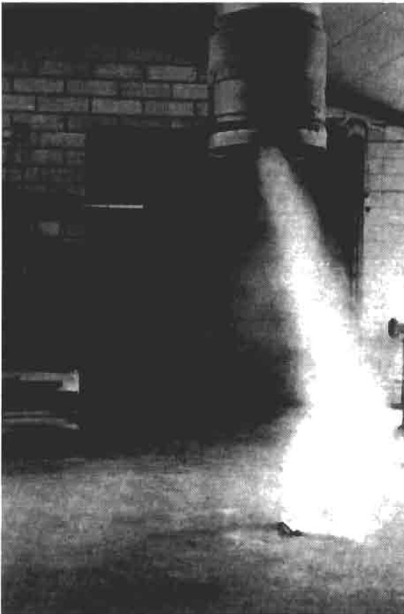
FIGURE 10.80 A typical Aaberg ventilator unit, which is suspended above the floor while smoke is released on the floor beneath the ventilator.
