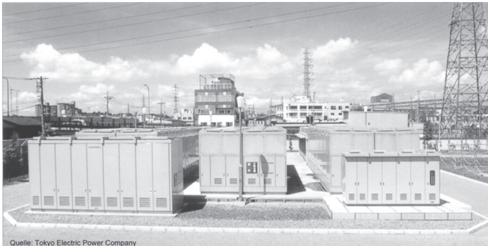
Fig. 10.13. Sodium sulphur (NaS) high temperature battery for load-levelling with 6 MW, 48 MWh (Tokyo Electric Power Company, Tsunashima).
