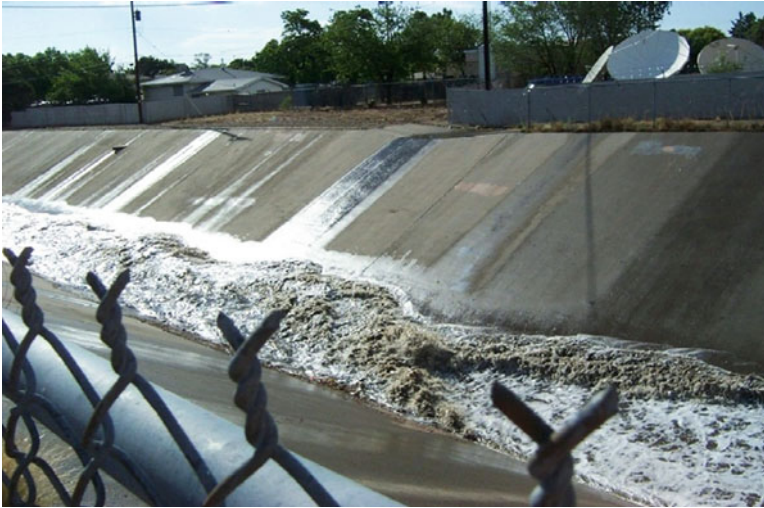
Fig. 2.4. Simple hydraulic jump occurring in a flood mitigation channel in Albuquerque, New Mexico, USA (Photo courtesy of Albuquerque Metropolitan Arroyo Flood Control Authority).
