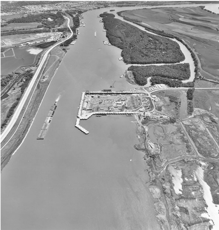
Fig. 6.13. Aerial view of the Mississippi River Lock and Dam No. 26 Replacement Project construction site near St. Louis, Missouri.
