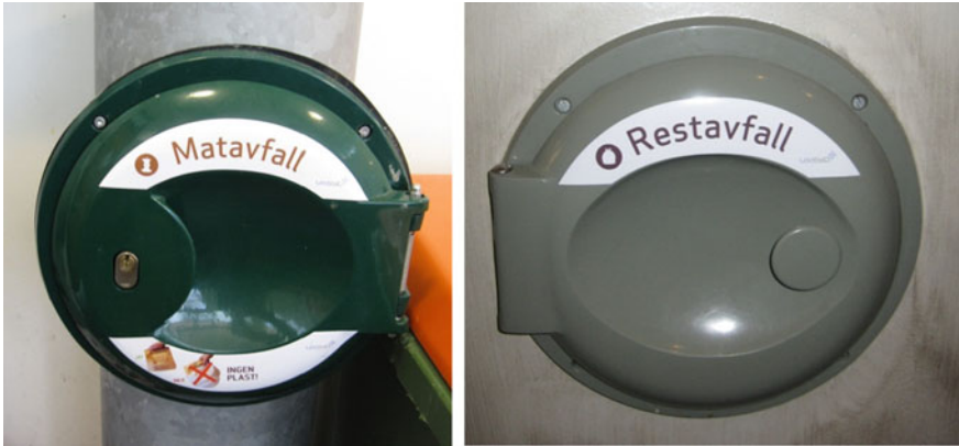
Fig. 4.4 Inlet doors for disposal of separately collected food waste in paper bags—with lock ( left ), and residual waste ( right ). Photo Maria Hoppe
