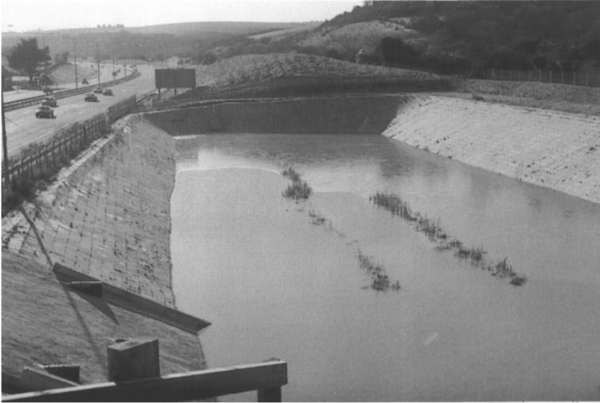
Figure 10.9 There can be no excuse for the ugly and anti-ecological character of most detention basins.
