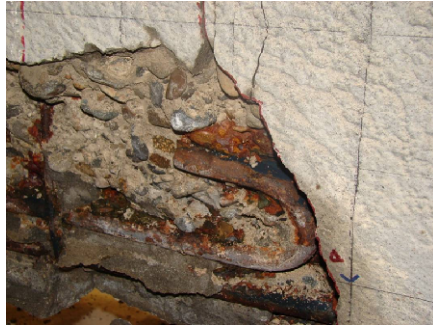
Figure 12. Exposed lap splice (Inner beam)
