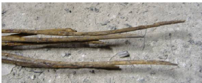
Figure 4. Example of failed wires in a prestressing strand in contact with the whitish segregated grout
