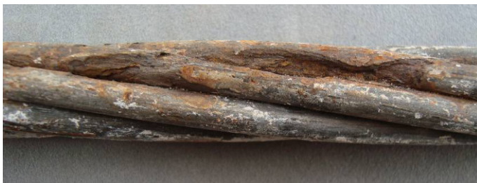
Figure 3. Example of corrosion attacks on a prestressing strand in contact with the whitish segregated grout
