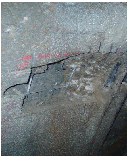
Figure 4: Detailed view of the place in which massive water penetration through the lining takes place. The new formations on the surface of lining are formed by calcium carbonate. These new formations are formed as the result of gradual “washing” of the concrete cement matrix.
