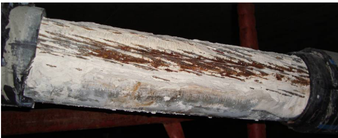
Figure 2. Example of whitish segregated grout embedding corroding strands
