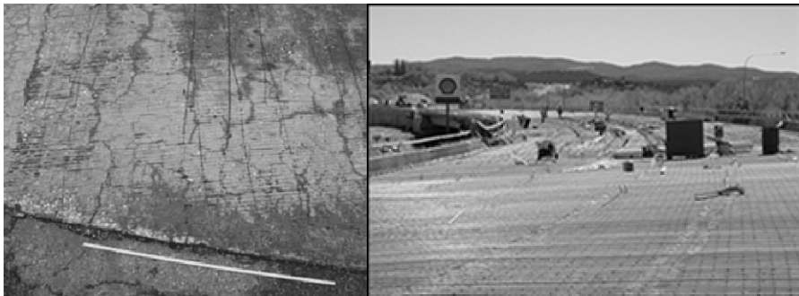
Figure 1. Crack on the Grinded Bridge Deck (left) and Scratched Epoxy-coating (right)
