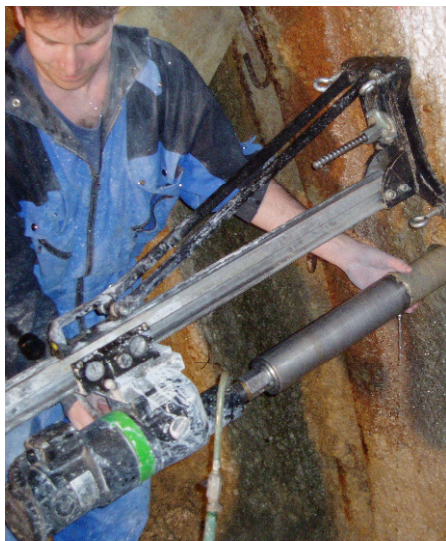
Figure 3: View of the locality in which intensive water penetration through the lining from sprayed concrete takes place.
