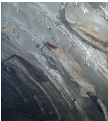
Figure 1: View of the locality where intensive water penetration through the lining from sprayed concrete takes place.
