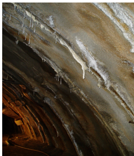
Figure 2: Detailed view of the place where massive penetration of water through the lining takes place. The new formations: on the surface of the lining are formed by calcium carbonate. These new formations are the result of successive “washing” of the concrete cement matrix .
