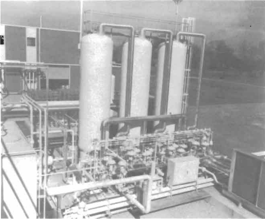
Figure 12-30. Molecular-sieve gas purification plant. Automated three-tower system removes carbon dioxide and water from natural gas prior to liquefaction. Courtesy of Memphis Gas, Light and Water Division
