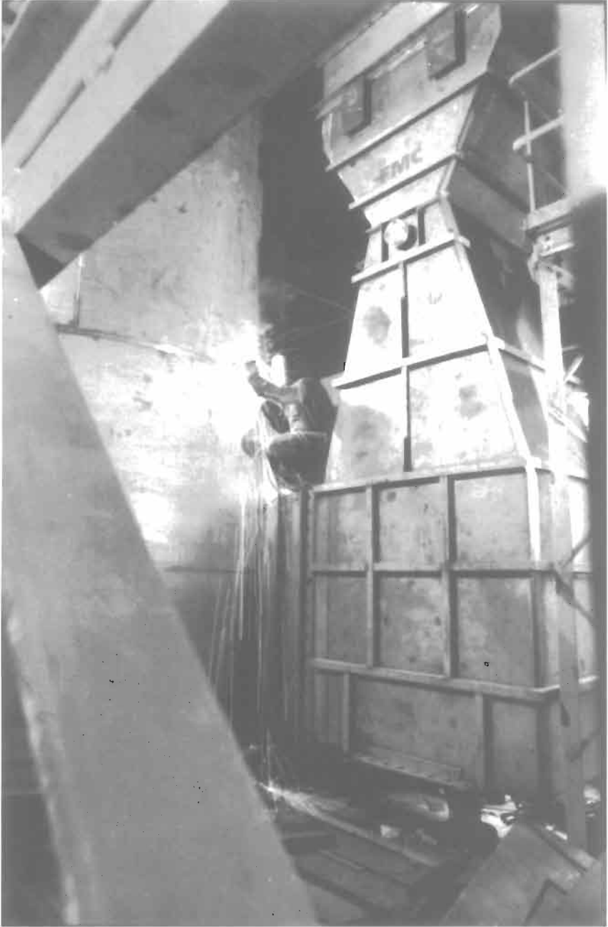
Figure 7-12. Venturi scrubber system being installed in a double alkali FGD plant. The unit shown handles 80,000 CFM of stack gas from the combustion of coal containing 3.2% sulfur. FMC Corporation
