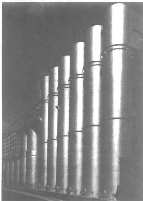
Figure 9-4. Manchester process plant treating 12 million scf/day of coal gas. Absorbers shown in foreground. Southwestern Gas Board, England, and W.C. Holmes Co., Ltd.
