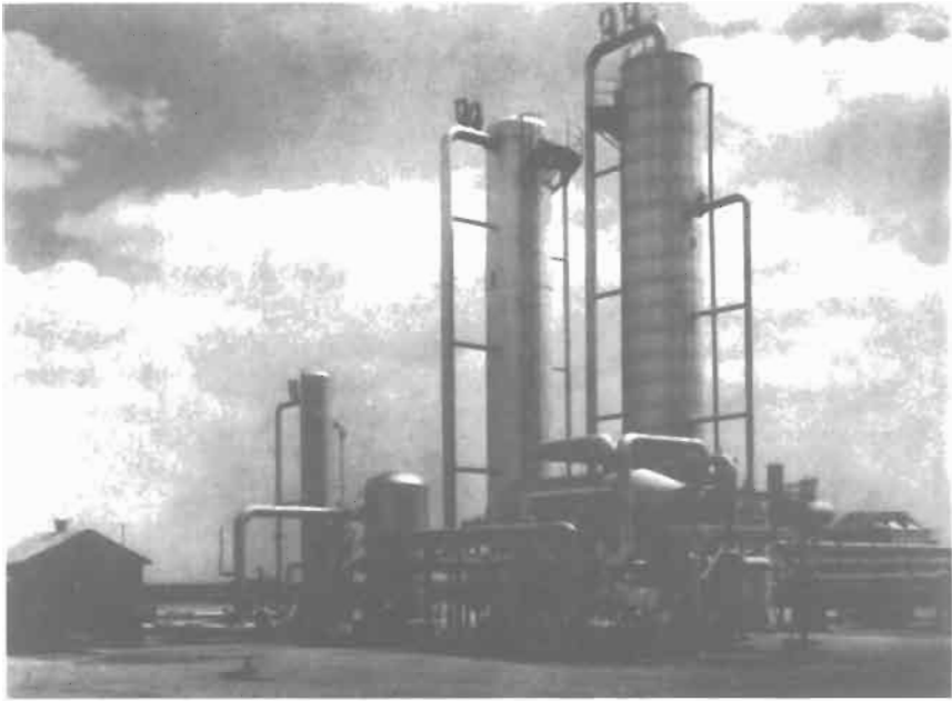
Figure 2-3. High-pressure gas-treating plant using Diglycolamine solution (Fluor Econamine process). Courtesy of Fluor Daniel
