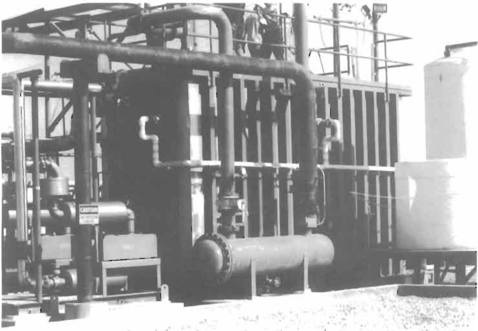
Figure 9-35. Oxidizer box and blowers on LO-CAT II plant at North Midway gas field, Bakersfield, CA. Courtesy of Wheelabrator Clean Air Systems
