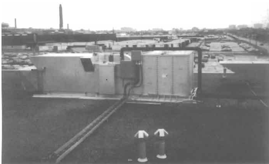
Figure 13-17. Ethylene oxide oxidation unit. Exhaust from sterilizer vacuum pump enters via black line on right. Courtesy of Donaldson Company, Inc.
