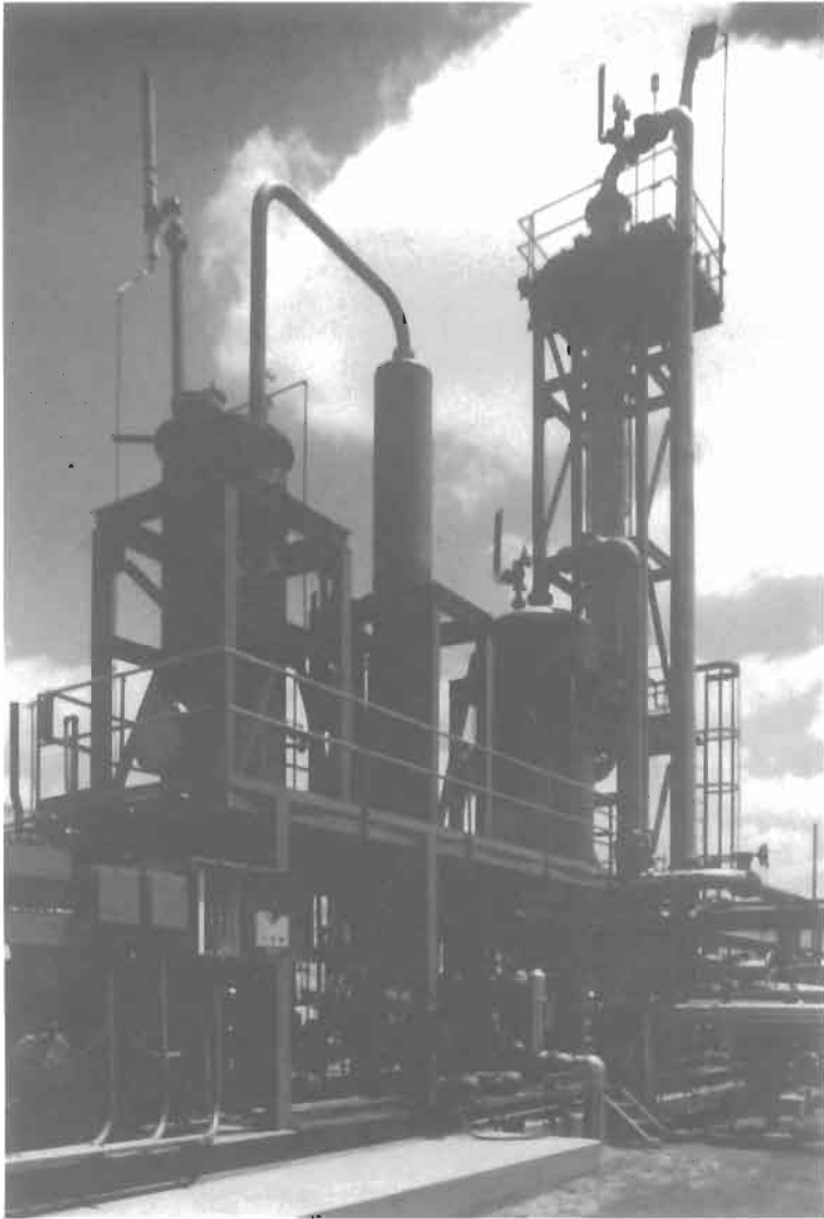
Figure 9-42. Photograph of 0.6 LTPD SulFerox plant with cocurrent downflow pipeline contactor. Courtesy of Dow Chemical
