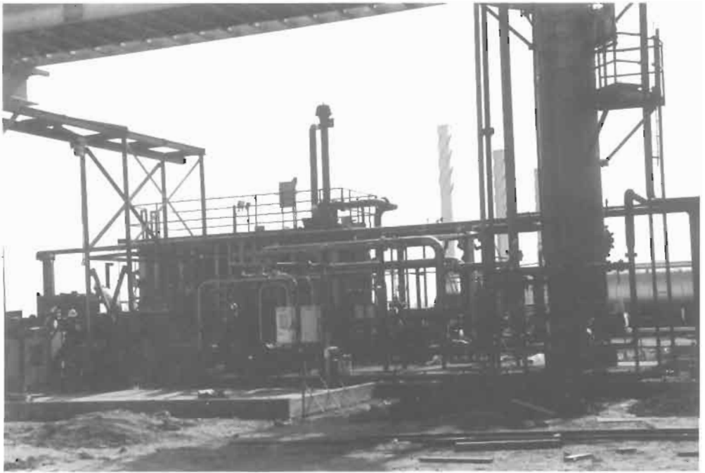
Figure 9-34. LO-CAT II equipment package at North Midway gas field, Bakersfield, CA. Courtesy Wheelabrator Clean Air Systems
