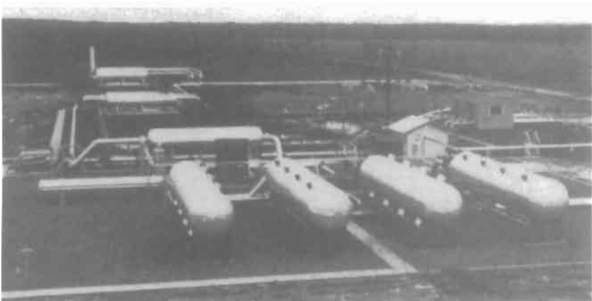
Figure 12-3. A large field installation for drying high-pressure natural gas with a solid desiccant. These adsorbers are of the horizontal compartmental type with four compartments per vessel. The gas is introduced through manifolds inside the units to provide even distribution. Regeneration gas is heated in a salt-bath indirect-fired heater. Courtesy of Black, Sivalls & Bryson, Inc.
