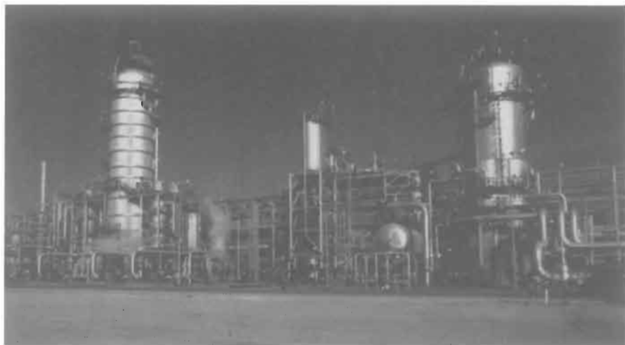
Figure 2-2b. Individual 540 MMscfd Improved Econamine gas treating train at Shedgum, Saudi Arabia. Contactor on right, regenerator with four vertical therosyphon reboilers on left. Courtesy Fluor Daniel
