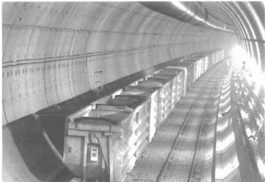
Figure 16.2 Use of precast lining segments in the UK north landward running tunnel of the Channel Tunnel showing spoil wagons running on temporary tracks (from Wilson, 1991).
