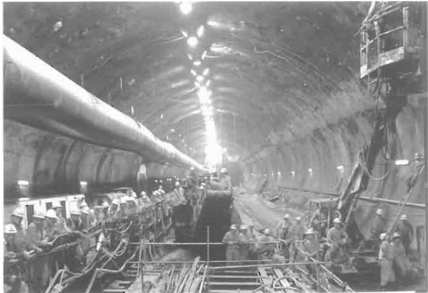
Figure 16.1 Workers awaiting the breakthrough of the south seaward running tunnel TBM into the UK undersea shotcreted crossover cavern in the Channel Tunnel (from Wilson, 1991).
