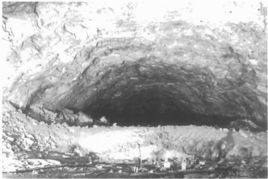
Figure 2.5 Construction of the underground facilities at the Alto Lindoso hydro-electric project in Portugal.
